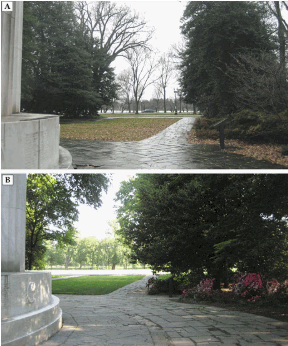
Figure 22. (a) View looking south past the memorial to Independence Avenue, illustrating the thick understory even in winter; (b) View looking north from the east side of the memorial (NCR CLP 2009). Note the broken flagstone paving in the foreground.
