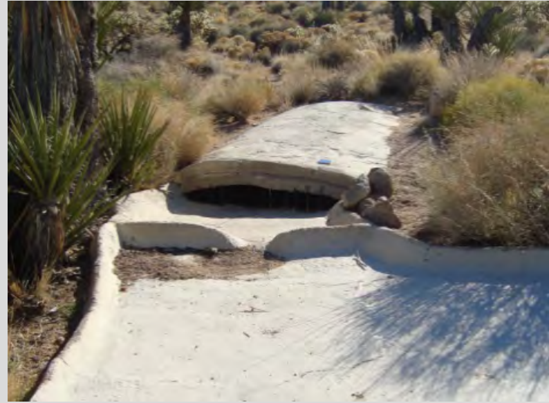
Small game guzzler with a concrete apron and underground tank
