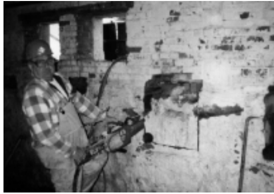
Figure 15. A hydraulic chain saw with industrial diamond teeth is being used to cut openings below the grade line for insertion of the steel beams.
