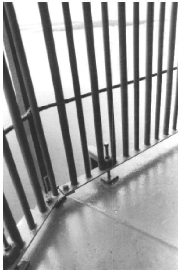
Figure 26. Note how the cage is clamped to the gallery deck, minimizing any impact on the structure's original fabric.
