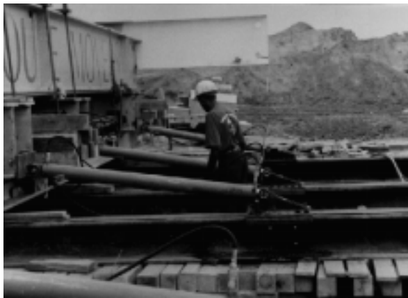
Figure 20. Four hydraulic rams set into the track steel pushed against the main steel to set the lighthouse in motion.
