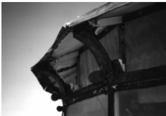
Figure 48. Reconstructing the cornice. The cornice plates were removed to expose the corroded cast-iron brackets and top channels. New brackets were cast in bronze, and the top sill channels were fabricated in stainless steel. Note the plywood ‘curtain’ erected for weather protection and shoring the lantern roof during reconstruction.
