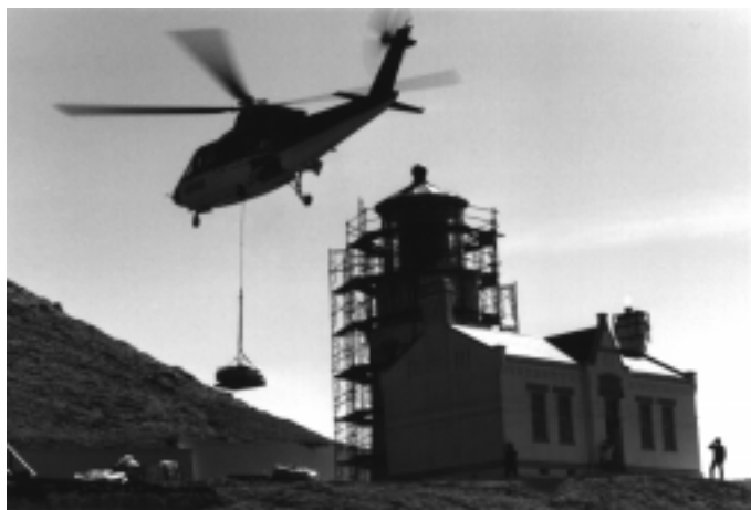
Figure 45. Staging the work. Note the temporary location of the auxiliary light on the fog signal building chimney.
