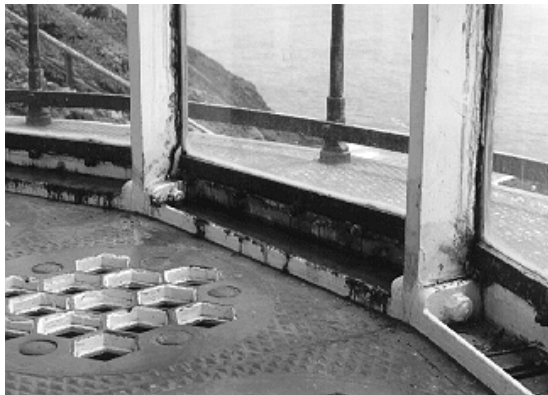
Figure 11. The water that has collected in this lantern sill is causing the iron lantern glass frame (the vertical members in the center of the photo) to rust and corrode.
