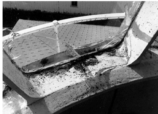
Figure 12. The glass in this lantern has been cracked by the rust-jacking that is occurring along the iron frame.
