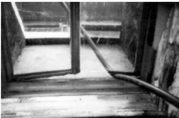
Figure 12. Close-up of severely deteriorated bottom rail of the same window in Figure 11. This condition can be repaired by splicing a new piece of sash
