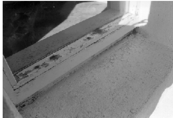
Figure 9. Rust occurring on the inside of the steel channel that forms the sill of this metal casement window.
