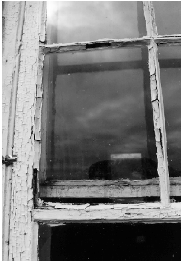
Figure 7. Deteriorated glazing putty and peeling paint on a multilite wood sash.
