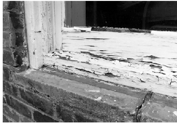
Figure 8. Deterioration of the bottom rail and sill on a wooden double-hung window.
