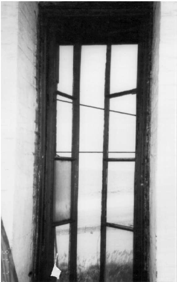
Figure 11. Example of a metal casement window in a lighthouse dating from the 1870s
