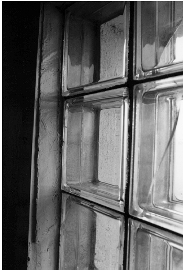
Figure 8. Close-up view of a glass-block window in a concrete lighthouse. The joint where the glass block meets the concrete wall should be caulked to prevent moisture infiltration.
