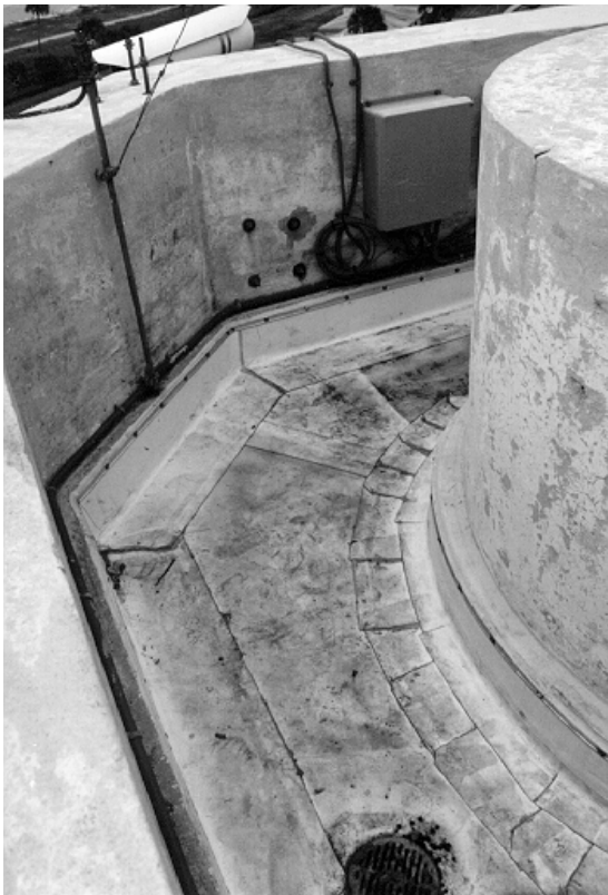
Figure 7. The concrete gallery deck on this concrete lighthouse has been covered with a rubber membrane. This covering should be checked regularly for leaks.
