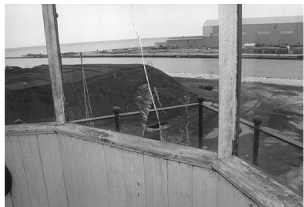
Figure 5. Storm glass with holes should be replaced as soon as possible to minimize water infiltration. If immediate replacement is not an option, the storm glass can be temporarily patched.
