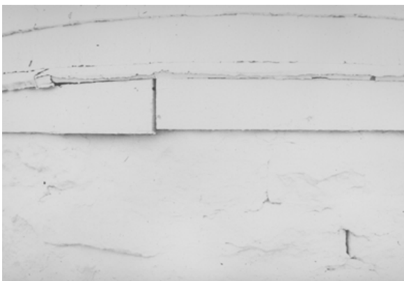
Figure 11. Open joints like those between these skirt boards must be properly primed, painted, and filled before mothballing the lighthouse.
