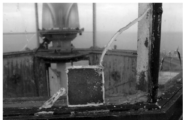
Figure 6. An acceptable temporary lantern glass repair made using a small piece of sheet metal and caulking.
