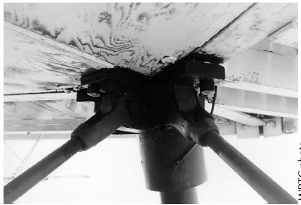
Figure 12. View of underside of a screwpile lighthouse. Although these bare wood surfaces are not directly exposed to rain, they are susceptible to mist and condensation moisture; and because there is no exposure to direct sunlight, the surfaces are seldom dry. For adequate protection during the mothballing period, these surfaces should be painted.
