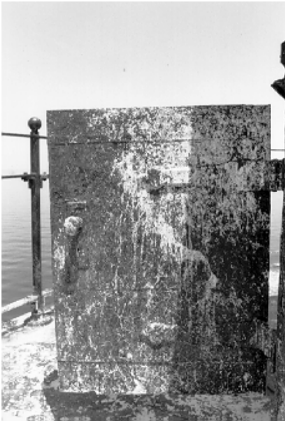
Figure 28. Surfaces such as this sheet-steel-covered parapet door that are covered with seagull guano should be thoroughly cleaned before mothballing and should be checked and cleaned once a year during the mothballing period.
