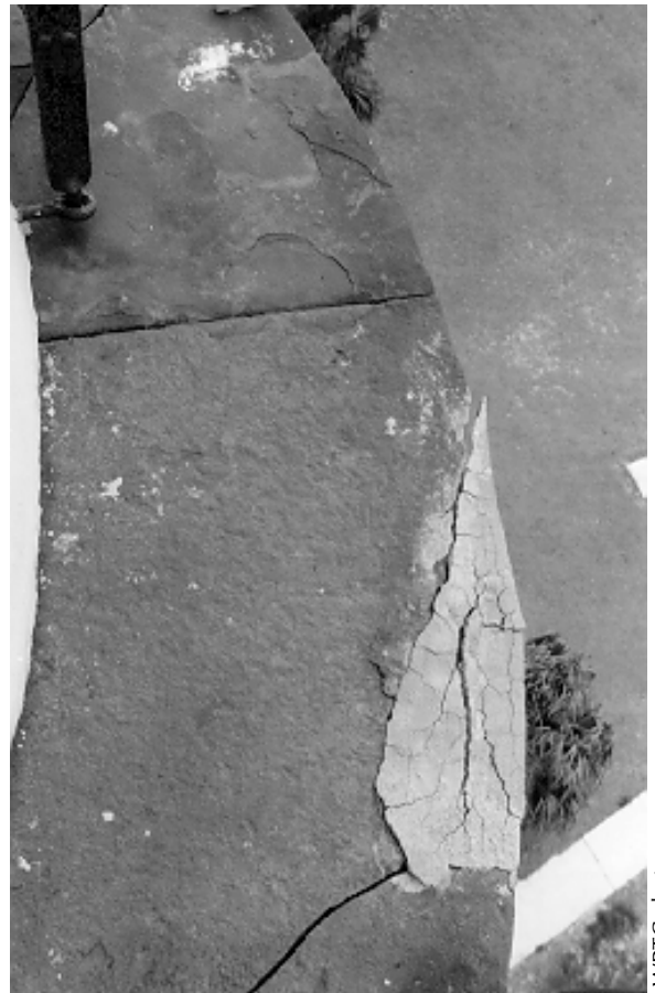
Figure 22. A failing repair made to a stone gallery deck using a simulated stone material. A stone dutchman repair should have been used.
