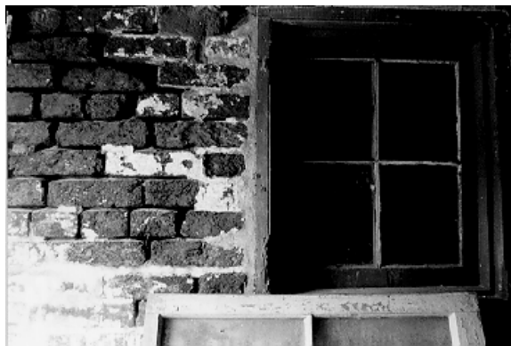
Figure 11. Detail of severely eroded brick and painting.
