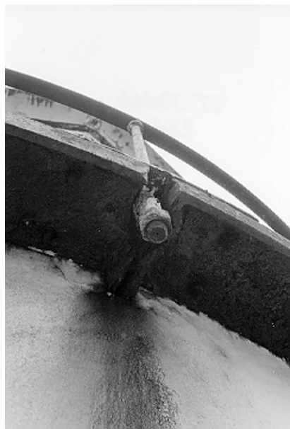
Figure 10. View of underside of gallery deck; the streaks on the stucco indicate that water is passing between the deck plates and possibly entering the masonry wall.
