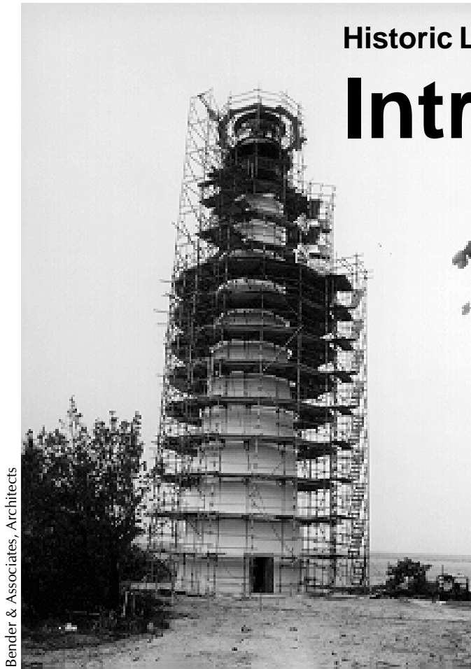
Figure 1. Brick replacement in 1996 restoration at Cape Florida Lighthouse on Key Biscayne, Florida.
