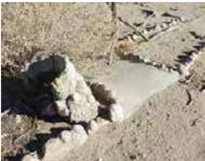
Figure 10.13. Bridge and broken planter at Block 35 Barracks 8 Apartment 1.
