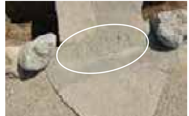
Figure 4.130. Detail of bridge at Block 15 Barracks 7 pond showing Japanese inscription in concrete.
