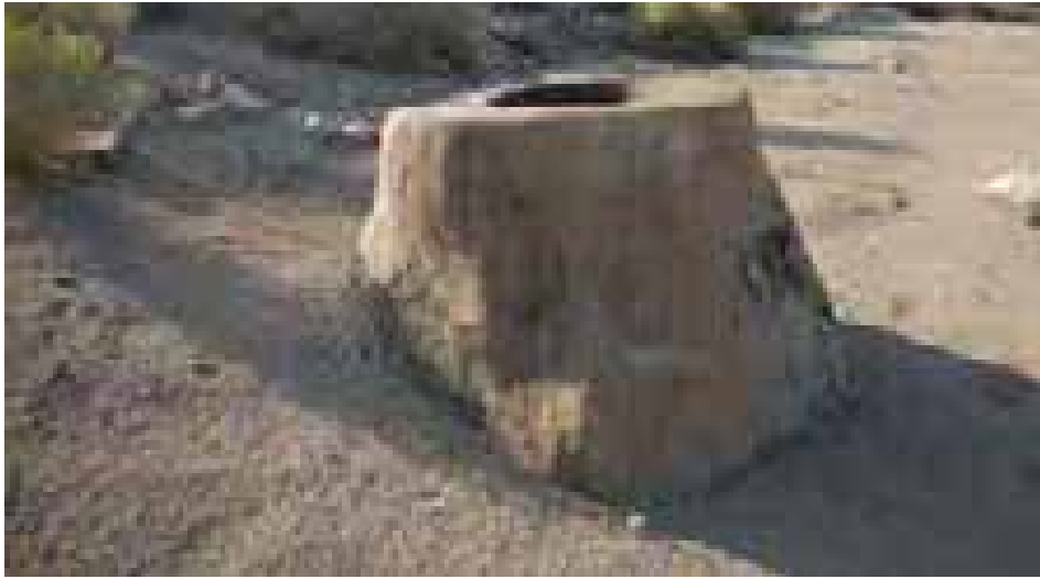
Figure 4.371. Faux-wood stump covering manhole at hospital.
