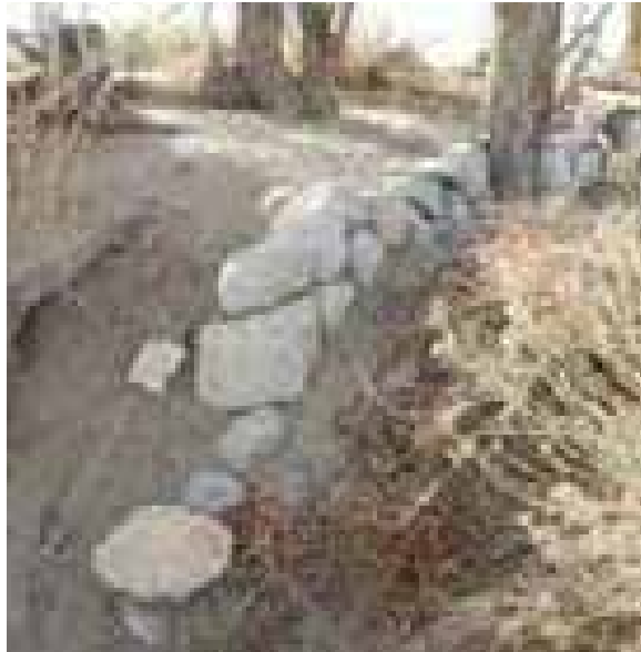
Figure 9.22. Breached rock retaining wall at hospital.
