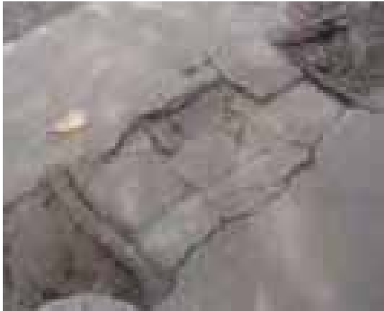
Figure 4.241. Broken concrete and wood bridge to Apartment 2 at Block 24 Barracks 5 garden.
