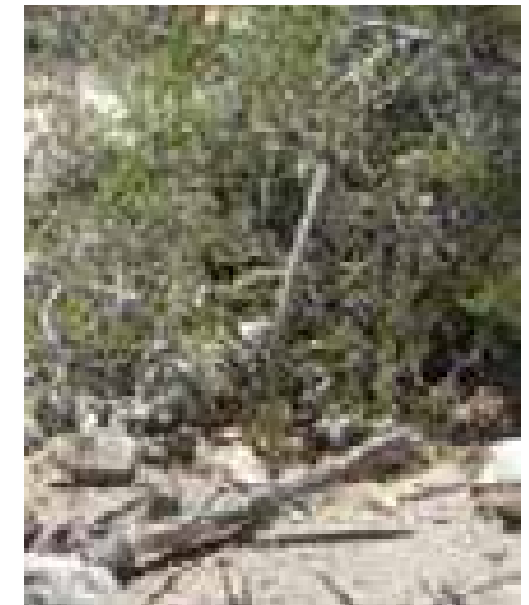
Figure 4.58. Vertical water pipe at Block 10 Barracks 13 garden.
