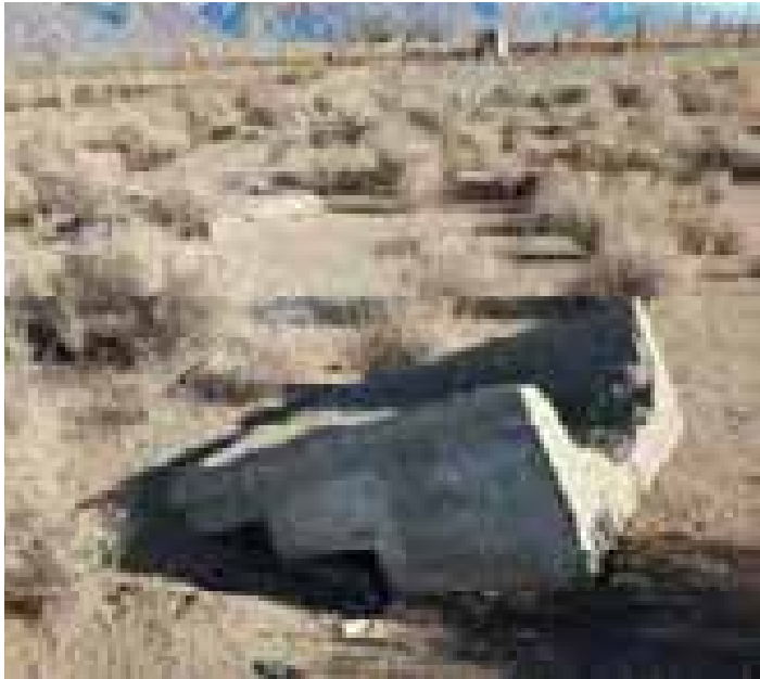
Figure 9.43. Overturned steps in administration area at Building L.
