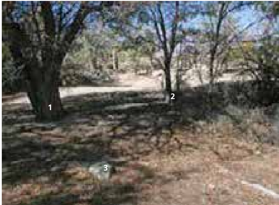
Figure 4.396. Trees (1 and 2) and rock (3) at upper pond at Merritt Park before excavation.
