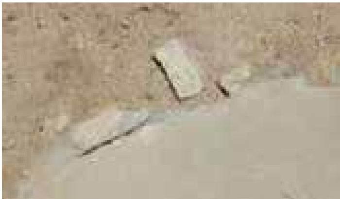
Figure 8.11. Broken concrete pond edge at Block 34 mess hall garden.
