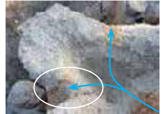
Figure 4.415. Detail of waterfall at Merritt Park showing added mortar and rocks to equalize water flow.
