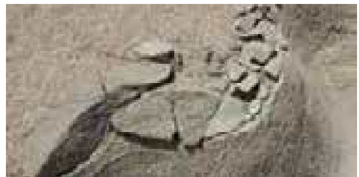
Figure 4.120. Block 15 Barracks 5 pond showing damaged concrete edge.
