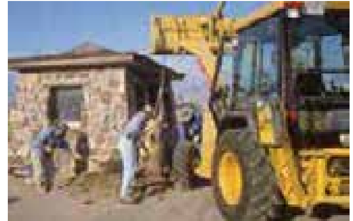
Figure 4.457. Replacing faux-wood stumps at military police sentry post (photograph by Charney White).
