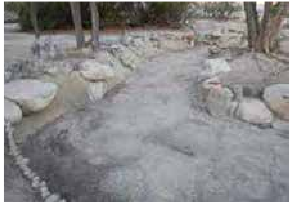
Figure 4.444. Upper pond at Merritt Park after repair of flood damage.
