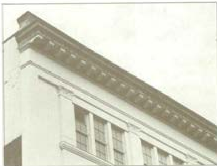
Sheet metal was often used for projecting cornices on commercial and industrial buildings. Cornices which have not been maintained can be replaced at moderate cost.
