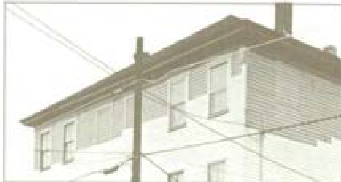
The application of synthetic siding can cause immediate or future damage to historic materials. The original window casings are being covered by vinyl siding.
