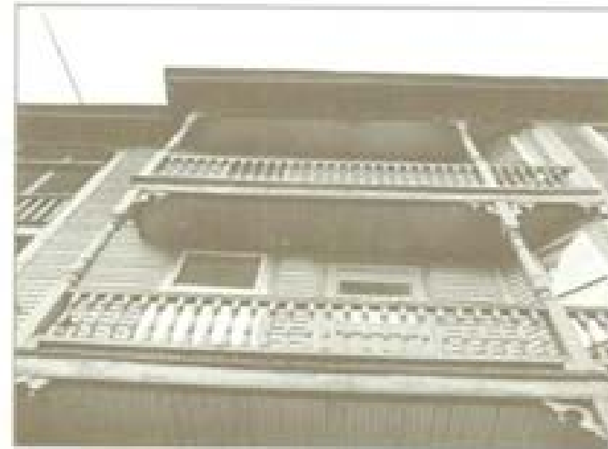
Original decorative architectural woodwork such as these characteristic triple-decker porches are often lost through neglect or attempts to "modernize" the building. This is detrimental to historic value.
