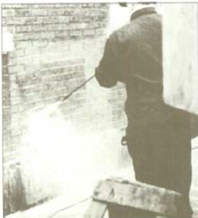
A cleaning test patch of the soiled masonry of the Gas Light Building will help determine the proper method for cleaning. Here the previously applied dilute acidic chemical is being pressure rinsed.
