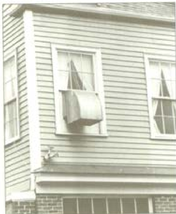
Intake and exhaust ducts and grilles are often necessary. Effort should be made to locate such features so that they do not detract, as in this case, from an historic facade.
