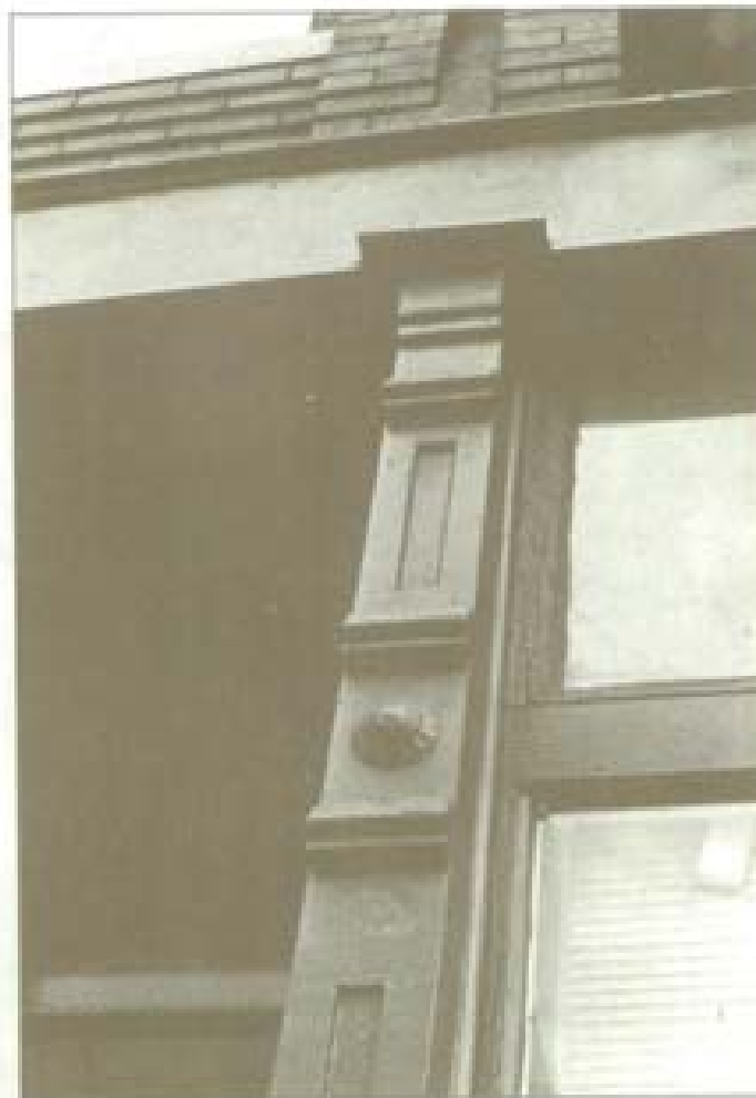
Buildings in Lowell, including the Union St. Joseph Building, pictured here. Whether or not covered by later remodelings, they are usually in perfect structural condition and need only repainting.
