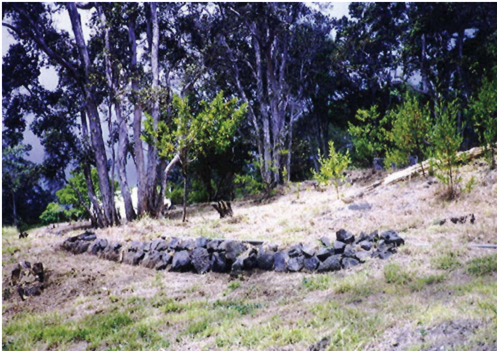
Buildings and Structures # 6: A dry-laid lava rock retaining wall located between the nursery area and the ranch house (PWR, HAVO, CLI files, 2003).
