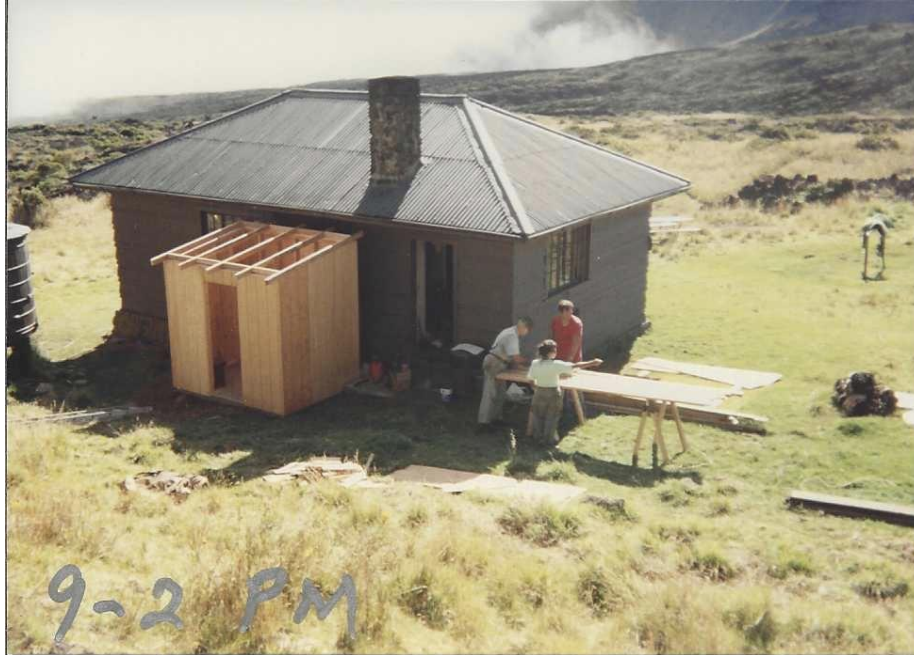
Hōlua visitor cabin shed, built by Andy Andersen Jr., Leif Andersen, Gloria Andersen, supervised by Ted Rodrigues
