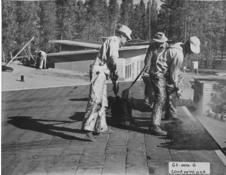
Fig. 1.3. Herbert Pownall. Built-up roofing system installation. 1953 Collection of Jackson Hole Historical Society, Folder 2003.0074, 2003.0074.029
