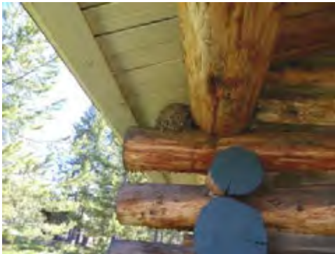
1. Bird's nest under soffit
