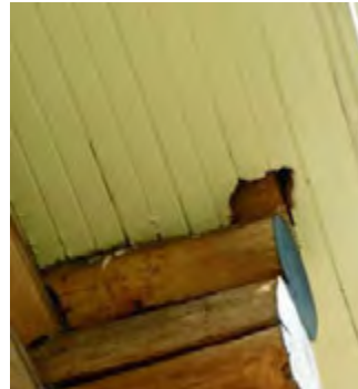
3. Holes in soffit provide animal access.
