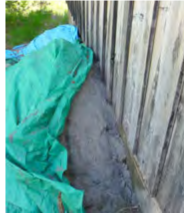
3. Sand piled against east wall
