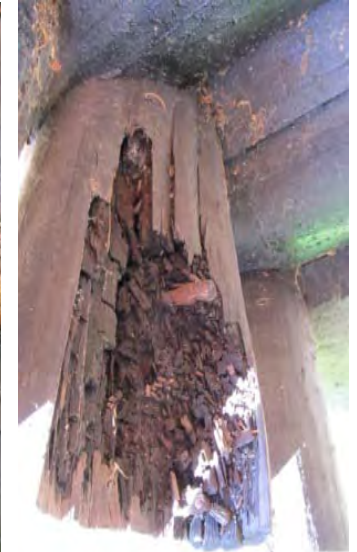
Water dripping on logs causes rot and deterioration.
