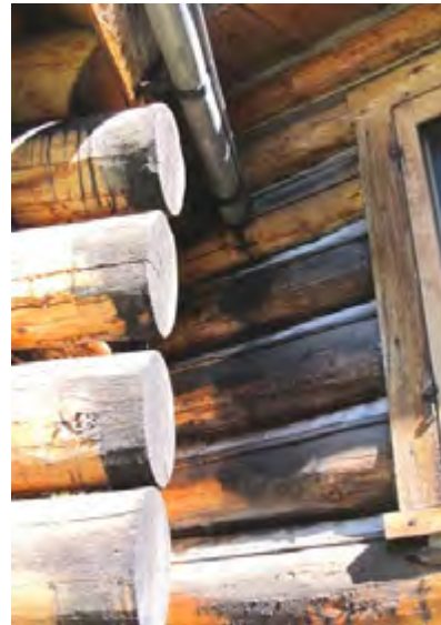
Water is dripping down wall instead of gutter causing black fungal growth on log
