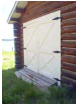
2. Ramp deteriorating due to poor drainage.
