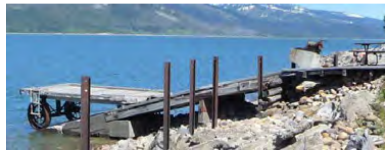
3. Foundation of the boat ramp is eroding.
