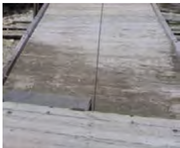
1. Aging and deteriorating planks.
