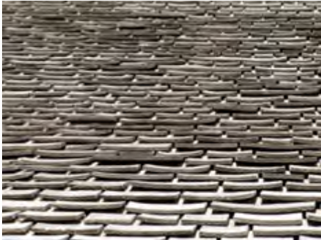
1. Curling shingles due to moisture retention on underside.
