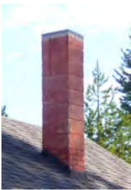
1. Chimney lacks metal flashing.
