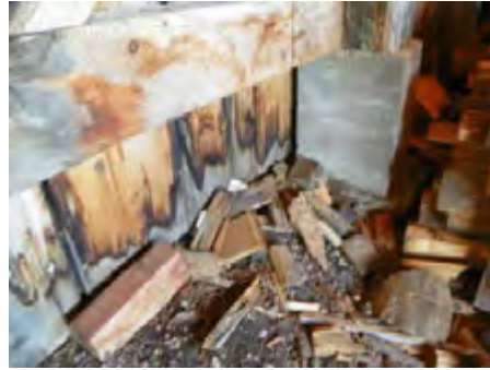
2. Build-up of dirt and scraps, west wall (interior)
