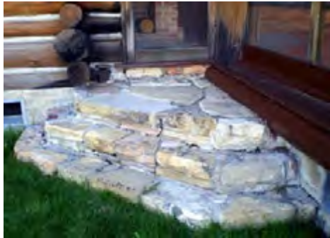
1. Sloping porch with loose stones
