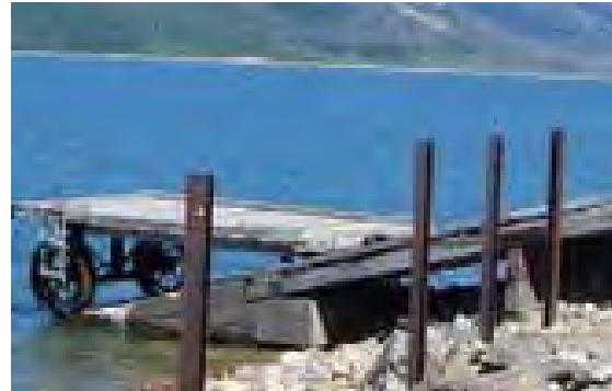
3. Erosion is undermining the boat ramp.
