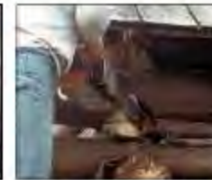
Remove Deteriorated Crown
