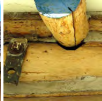
3. Log does not fit into notch.
