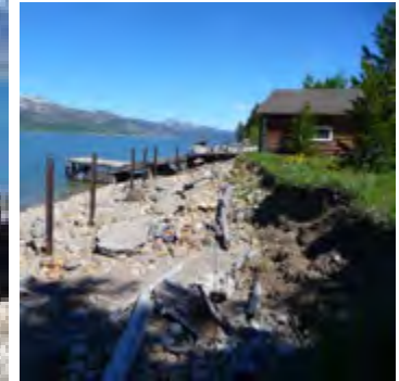
4. Overall, the sea wall is an important issue.
