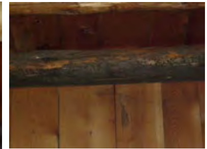
5. Ridgepole in main room is stained with fungus, indicating moisture control issues.
