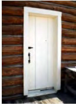
1. Missing door sill.
