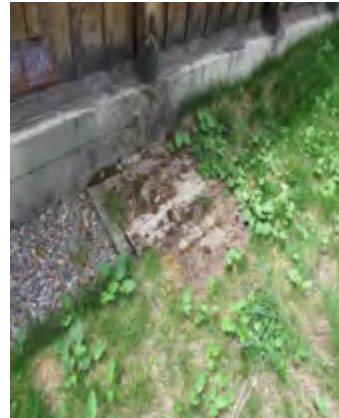
Wooden crawl space door where water drains underneath building
