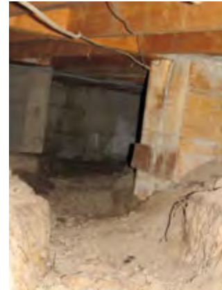
Trench under building where water drains causing mold on foundation
