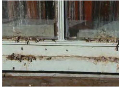
3. Bird droppings on window sills hold moisture and cause decay.
