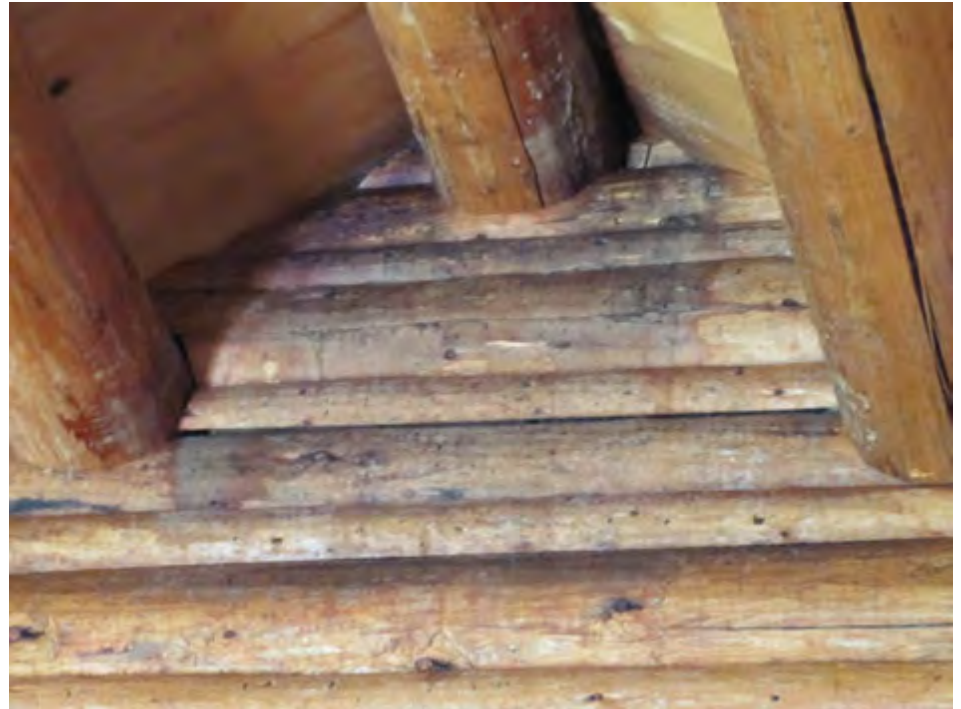
Damage to the upper logs in the Berol Lodge living room.
