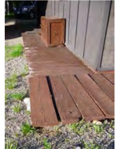
2. Loose porch decking, NW corner
