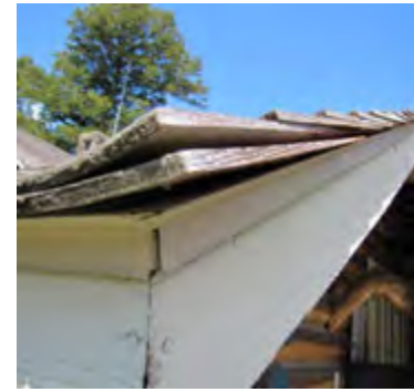
3. Shingles bowing due to moisture absorption.
