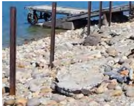
2. Rip-rap is nonfunctional.
