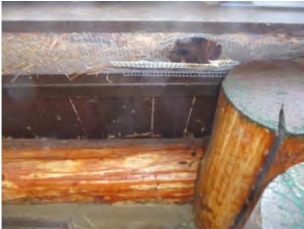
1. Screened soffit vent has numerous holes.
