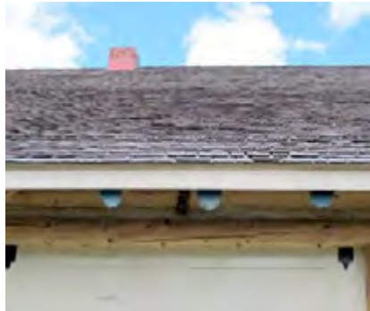
2. Roof sways at middle of west elevation.
