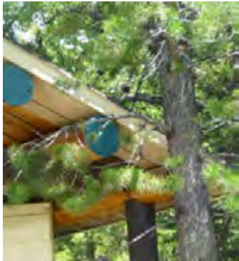
1. Trees are growing next to and over the roof.
