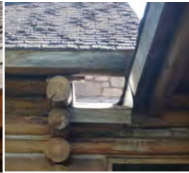
2. Large flashing trough promotes poor drainage
