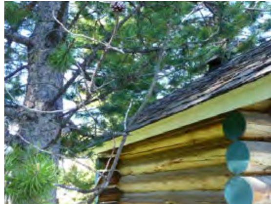
2. Tree at SW corner of roof
