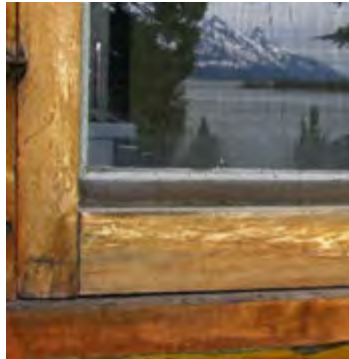
2. Window collecting debris; sill finish and glazing deteriorating
