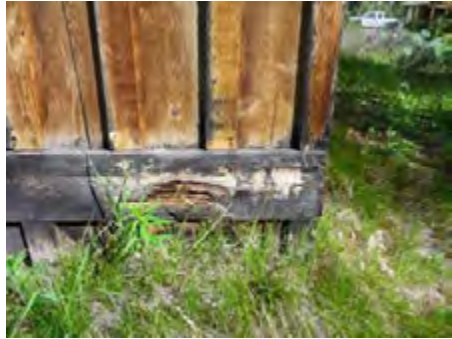
1. Fungus and rot at northwest corner
