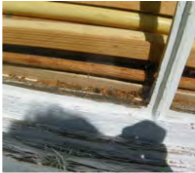
1. Paint peeling and debris accumulating in window sill.
