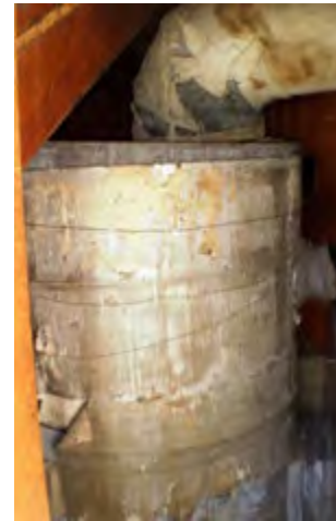
4. Boiler and pipes are wrapped in asbestos.
