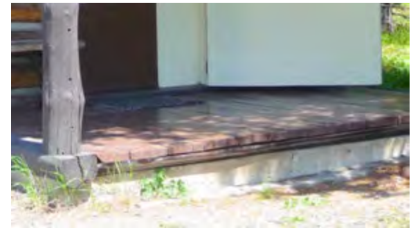
3. Porch decking boards loose.
