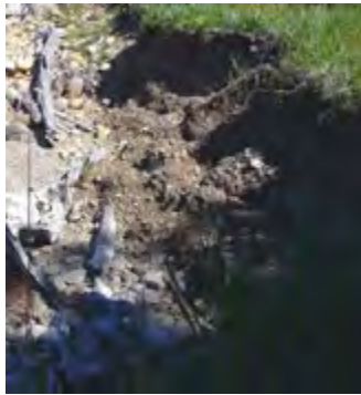
1. The shoreline is eroding.
