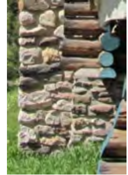
4. Stone repairs improperly done.
