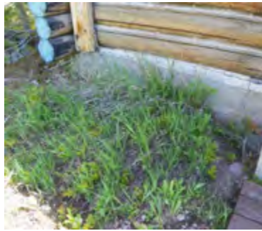
2. Foundation is cracked; vegetation close to building.
