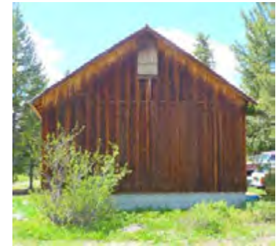
4. Vegetation too close
