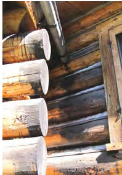
Water is dripping down wall instead of gutter causing black fungal growth on log
