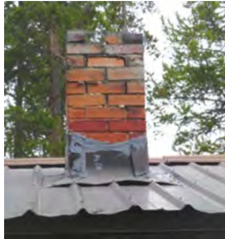
2. Incorrect chimney flashing and pointing
