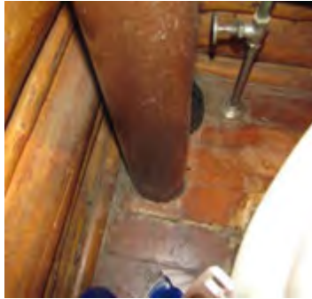
2. Water damage in the bathrooms.
