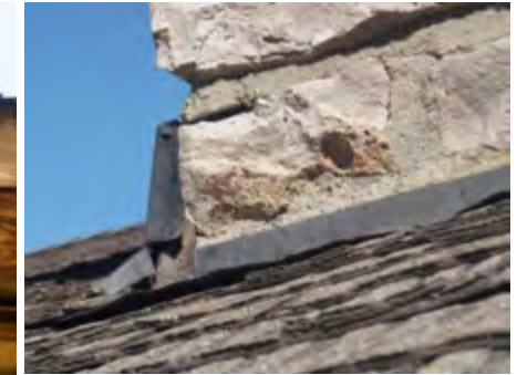
4. Gaps in flashing around chimney
