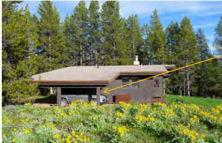
1. 40+-year-old built-up roof
