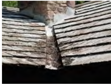
2. Flashing in valley is not correct.
