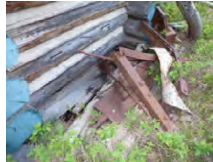
3. Equipment leaning on building
