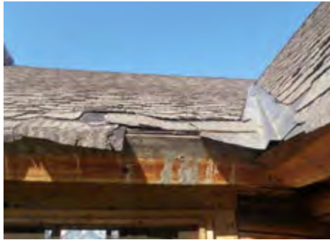
1. Drooping shingle edge and valley flashing
