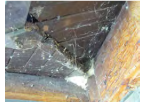
4. Soffit is warped in corner due to poor flashing above.
