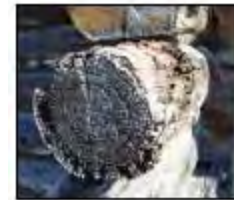
Deteriorated Condition (CWA)
