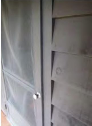
1. Screen door does not close.
