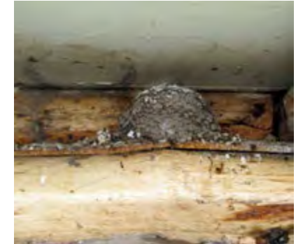
4. Swallow nests are being built under the eaves.
