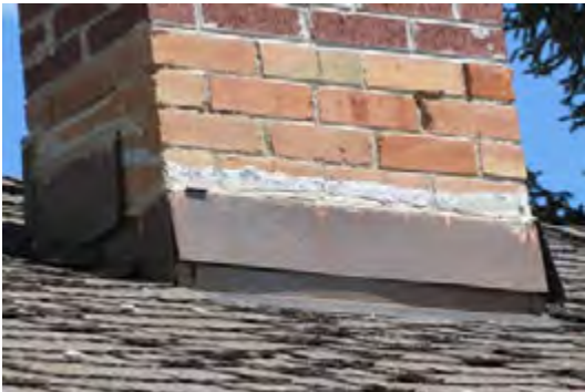
1. Flashing on chimneys should be properly tied into the roof.
