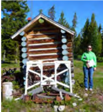
1. Building leaning to west
