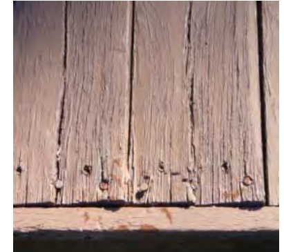
4. Porch decking boards loose.
