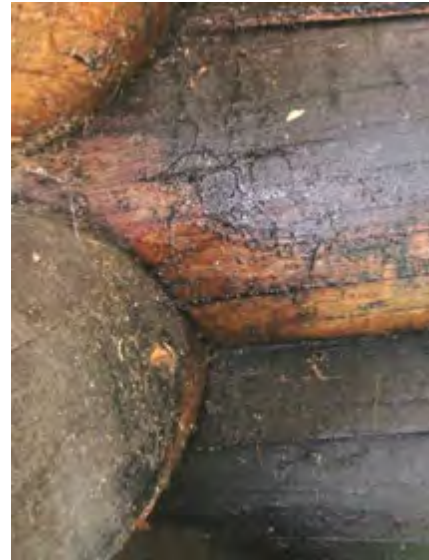
Corner has lots of black fungal growth and is constantly moist.
