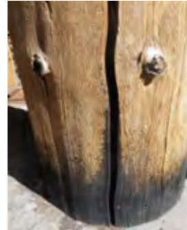
3. Porch column discolored and infested
