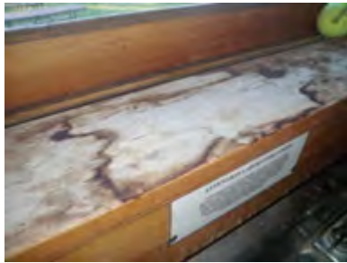
1. Interior window sills experiencing water damage.
