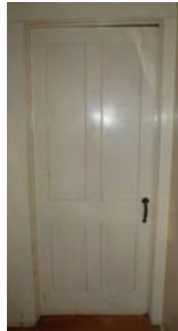
3. Doors are out of alignment.
