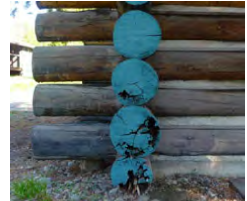
3. Rotted log crowns, NE corner
