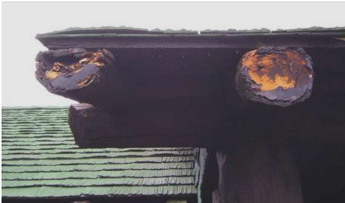
South elevation, wood decay on porch roof rafter tails
