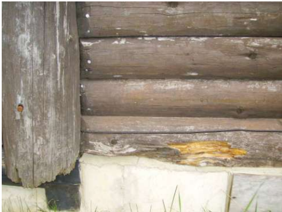
North elevation, sill log of middle enclosure used as darkroom and storage showing possible adverse animal activity
