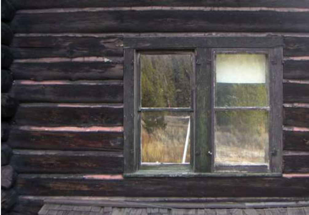
Figure 42 West wall of Rm. #5 with double hung windows (right window has a storm sash)
