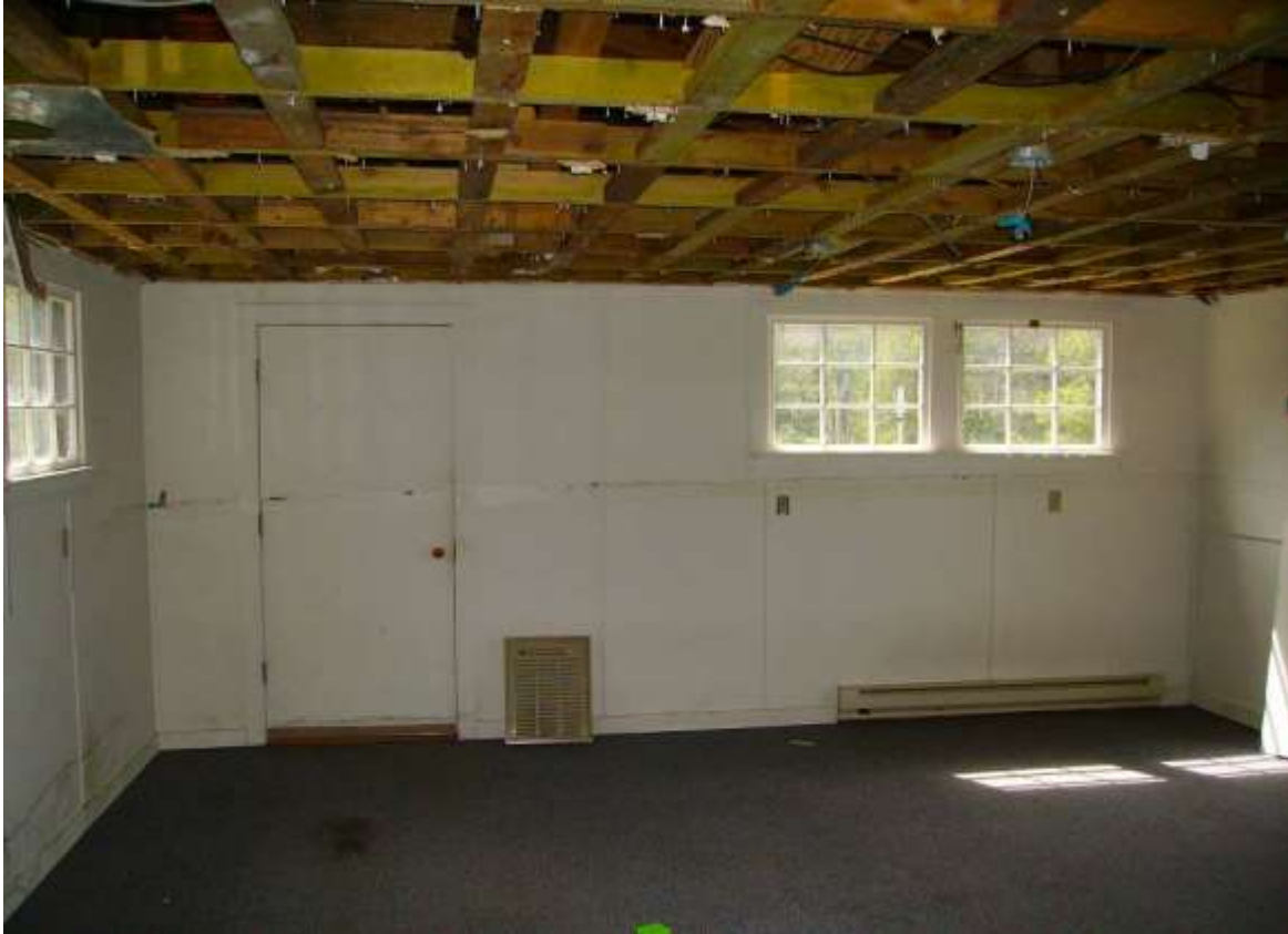
Figure 46 Interior of Rm. #9. Note interior use of pressure treated lumber in ceiling joists
