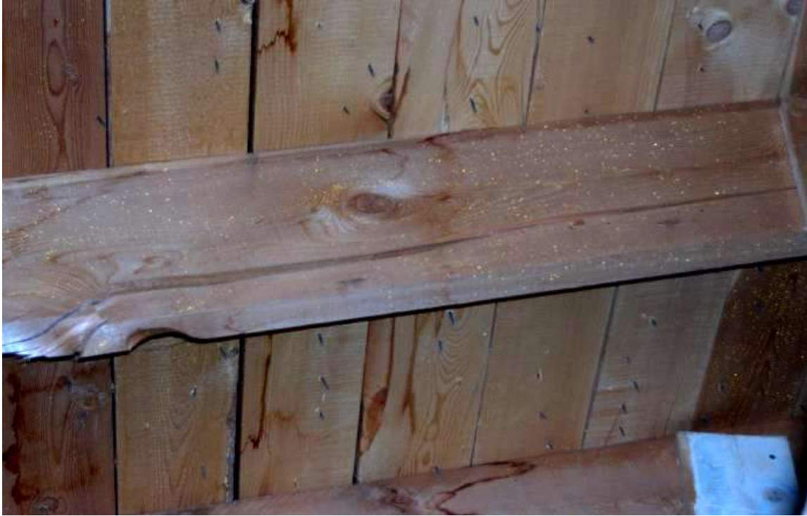
Figure 47 Cracked rafter in Rm. #9
