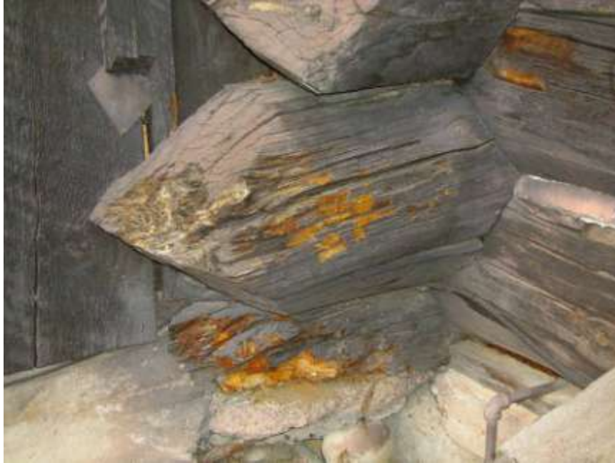
'Beaver tails' at junction of 1956 addition with CCC west addition showing foundation and tail decay; note metal patch blocking rodent entry
