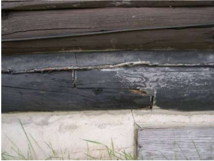
North elevation, splice on earliest addition at foundation level, note covered vent on bottom right
