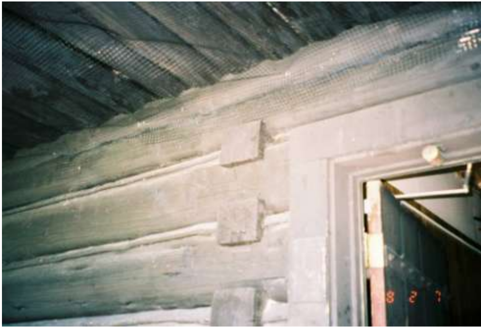
Typical wire netting used to block entry of rodents into the building
