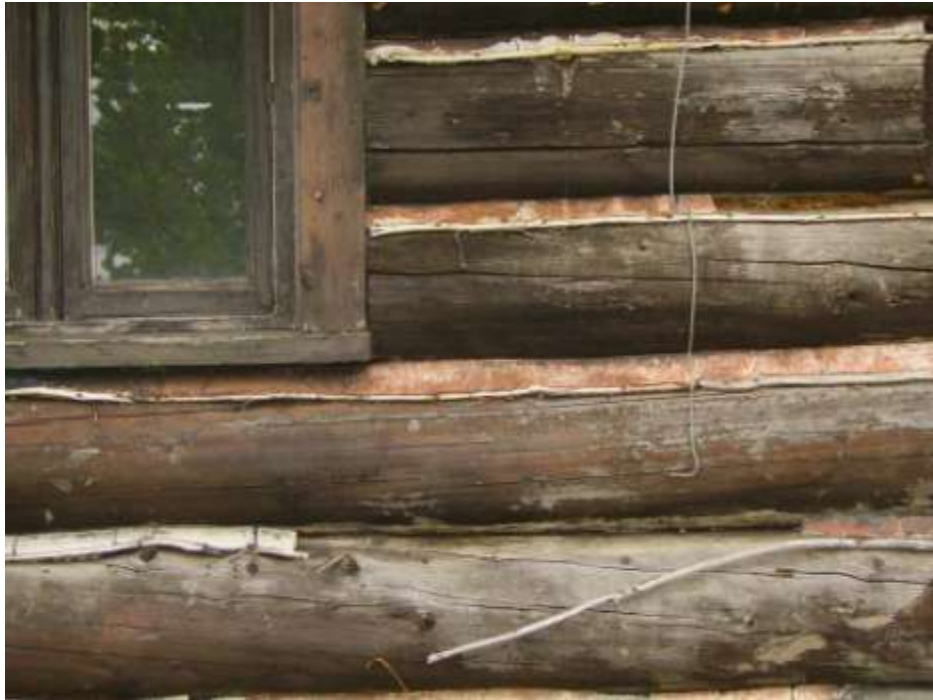
Chinking and daubing on north elevation showing need for replacement
