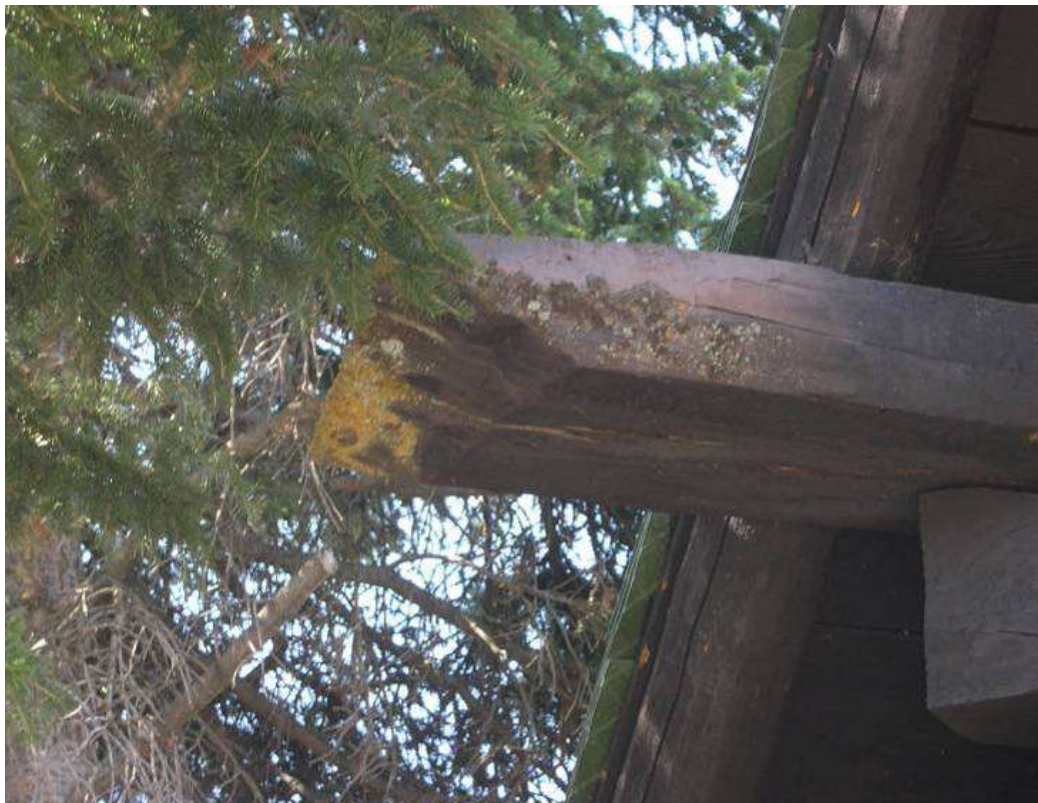
Figure 51 Exposed log tail deteriorating due to moist conditions related to tree as southeast corner of building
