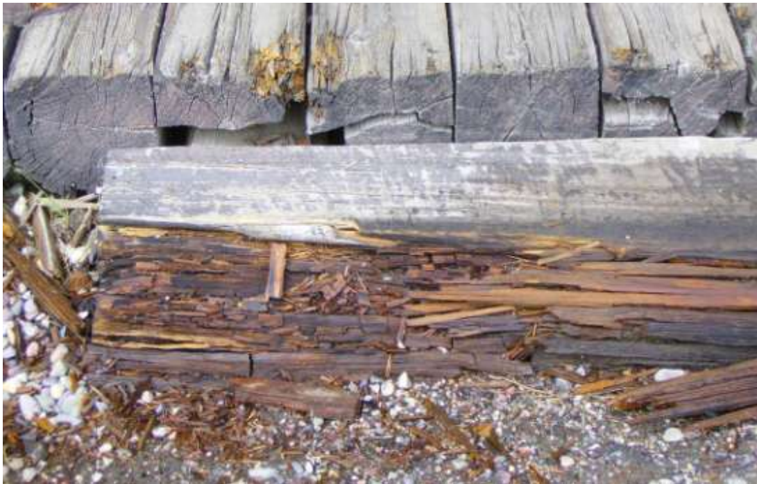
Entry step showing deterioration
