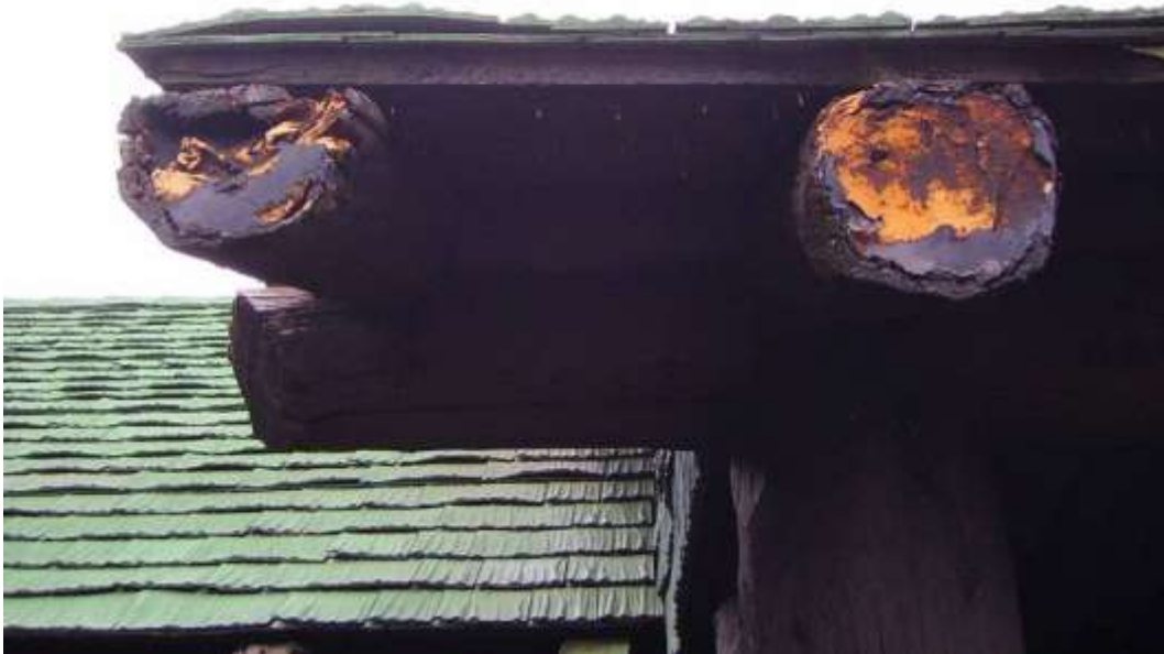
Figure 38 Wood decay at exposed porch rafters
