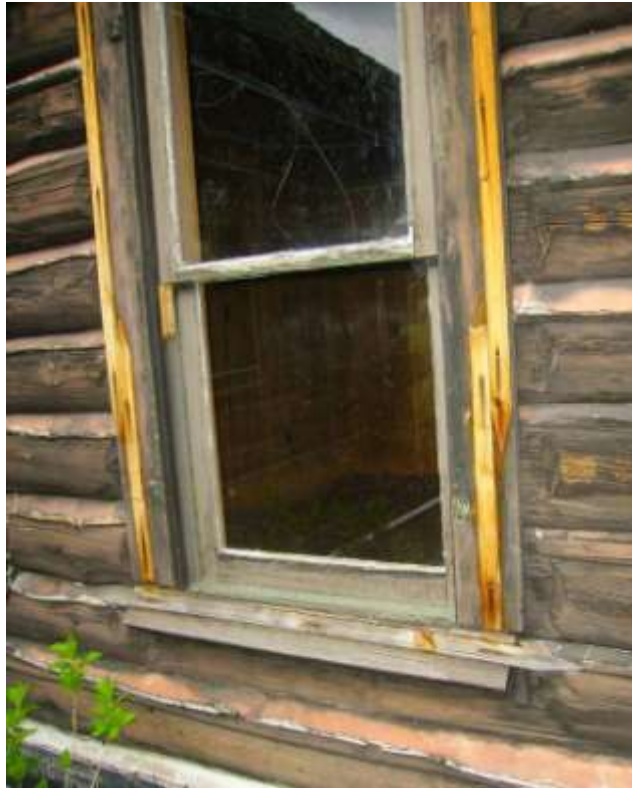
East elevation of earliest addition, showing scarring suggesting position of earlier window
