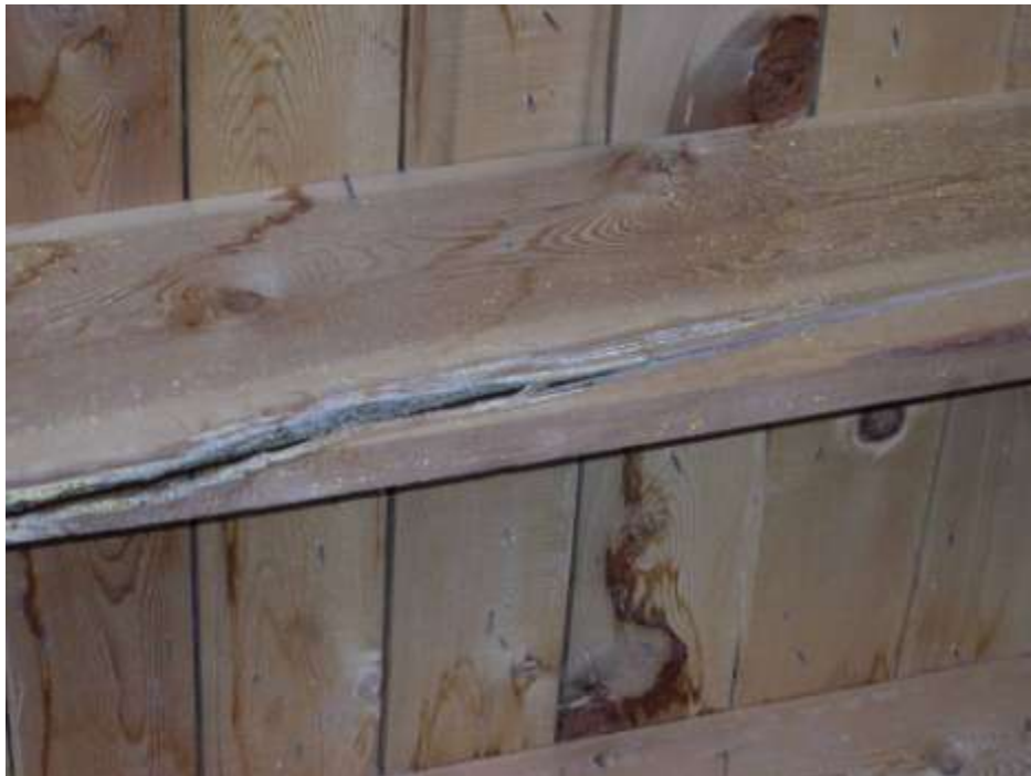
Ceiling of 1956 addition, showing major crack in rafter
