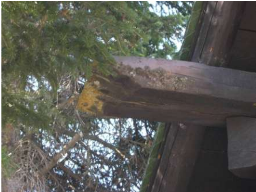
East elevation, decayed purlin on CCC addition
