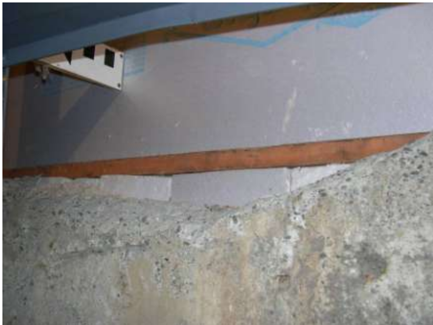
West interior basement access/egress, concrete sill showing wear; note sheet insulation at top of photo
