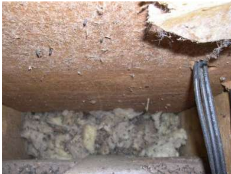
Figure 7 Void in wall in Rm. #4 where old chimney existed
