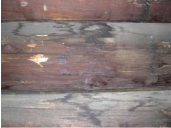
Typical evidence of exterior water damage
