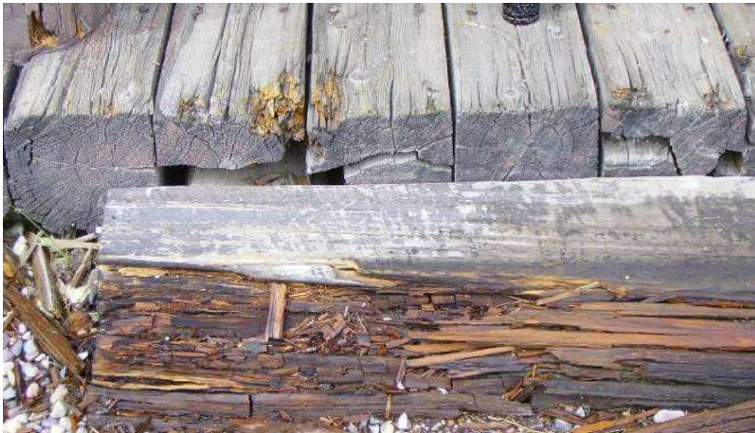
Figure 40 Decay of porch timber
