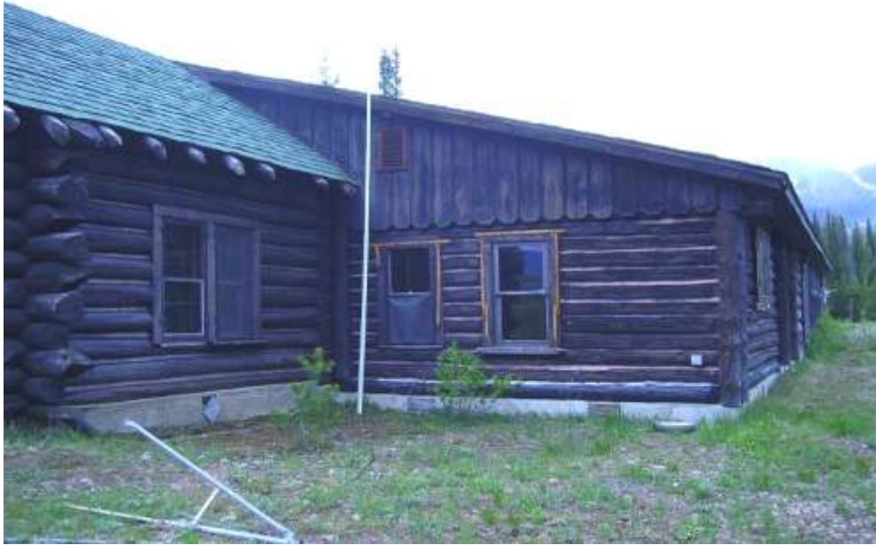
Figure 41 Shed roof as seen from the east. Note missing log rafter tail
