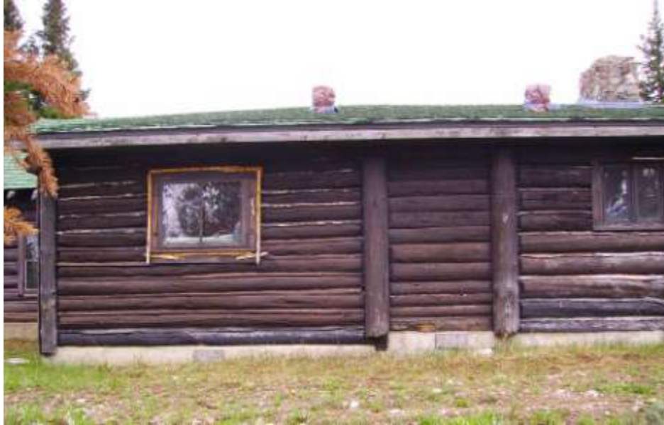
North elevation, light-colored lathe around window is left from weather film.
