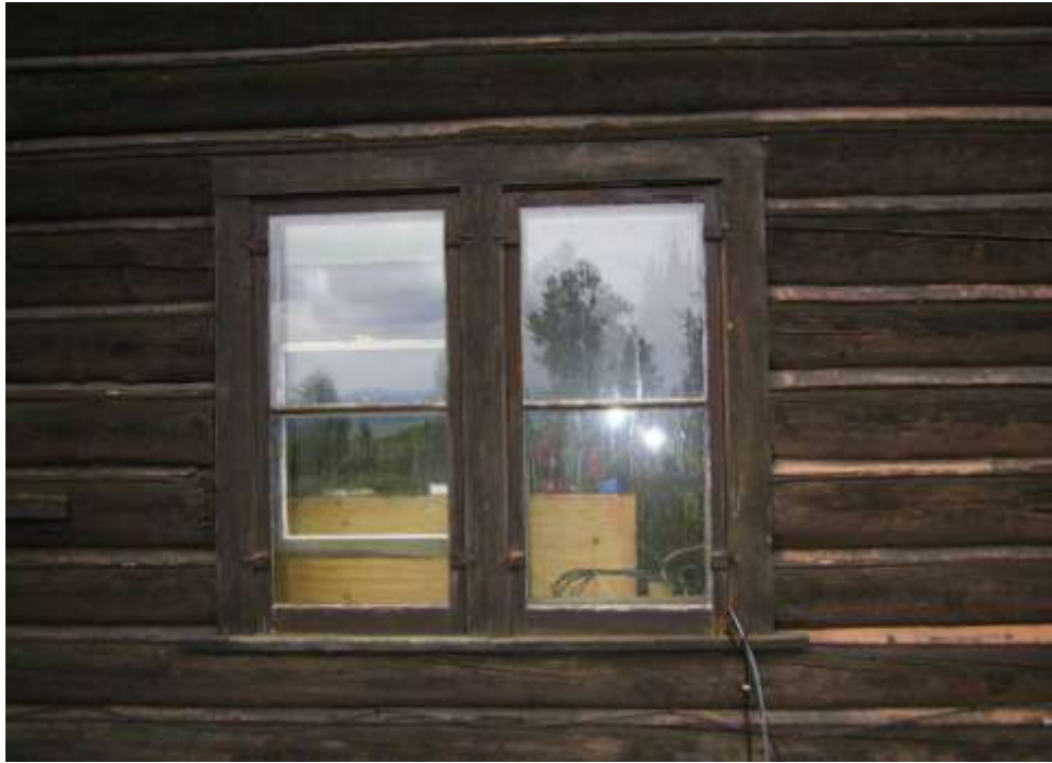
East elevation, CCC addition, windows, logs, chinking and daubing all in good condition
