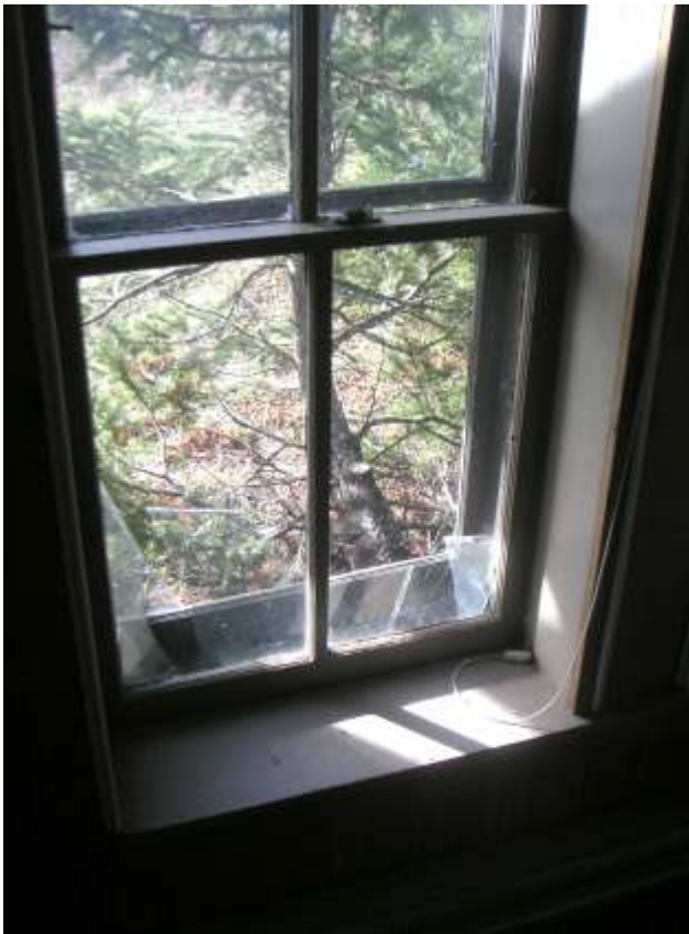
Figure 43 Double hung window with broken panes in storm sash
