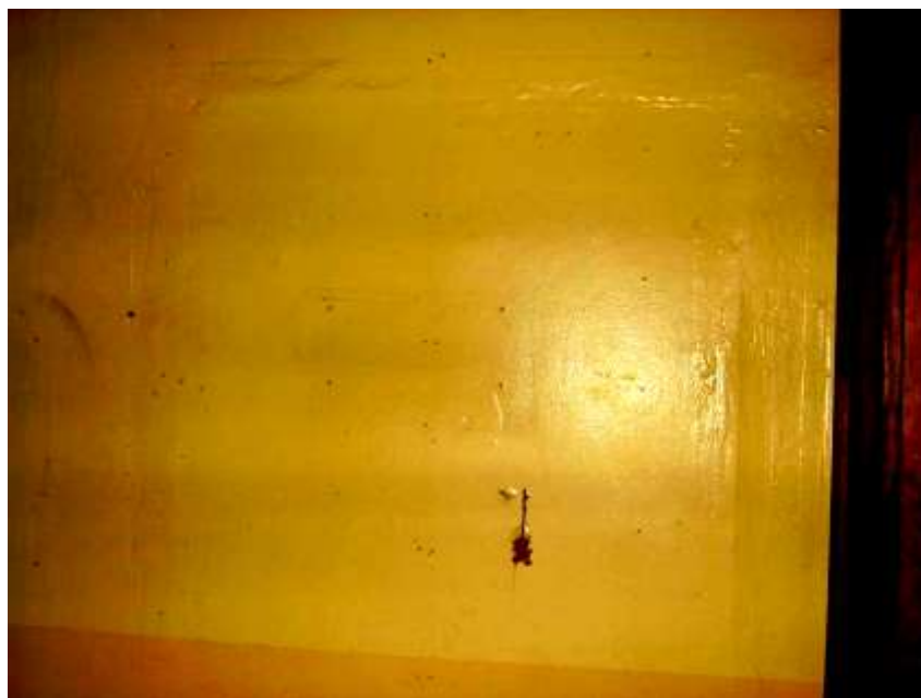
North wall of room #4, rake light showing perimeter of previous doorway to exterior wood shed (now bathroom)
