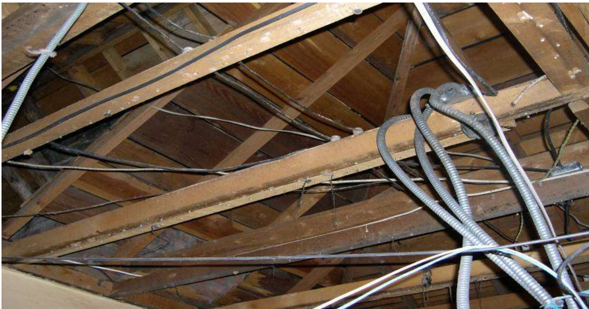
Figure 52 Various types of exposed electrical wiring
