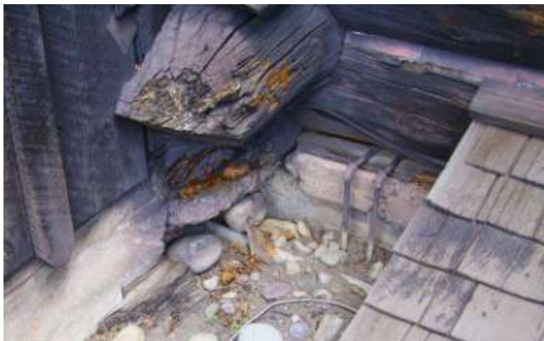
Figure 24 Log decay at corner of addition
