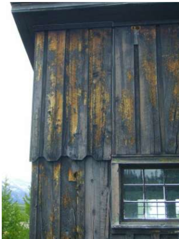
Southwest corner of 1956 addition showing deterioration likely due to weather
