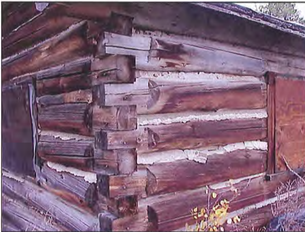
Figure 42. Detail of the corner notching and wall daubing in HS-1157, Cabin 12. Source: A&E Architects, 2004.
