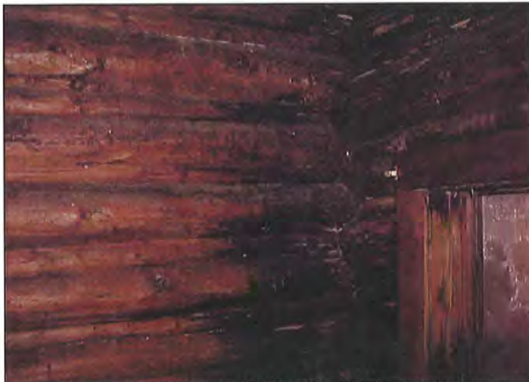
Figure 75. Interior wall showing water staining, HS-1163, Cabin 7. Source: A&E Architects, 2004.
