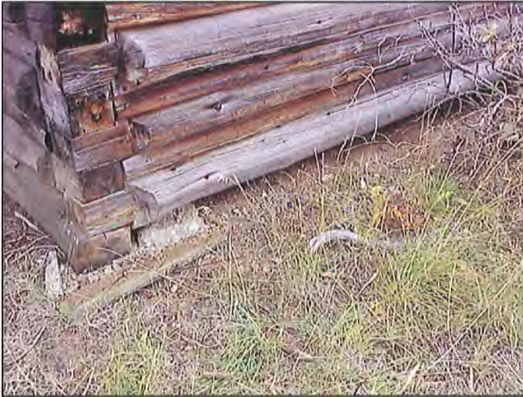
Figure 28. Detail of deteriorated foundation pier, HS-1155, Cabin 15. Source: A&E Architects, 2004.
