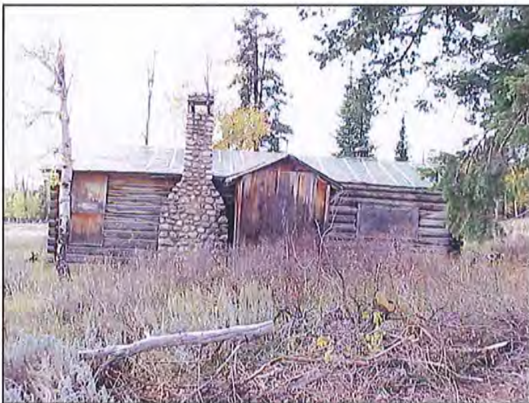
Figure 32. North wall of HS-1156, Hammond Cabin; the frame addition in the approximate middle of the wall contains a bathroom. Source: A&E Architects, 2004.
