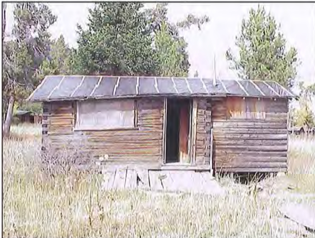
Figure 25. South wall of HS-1155, Cabin 15; bathroom addition to right. Source: A&E Architects, 2004.
