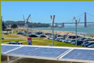
Solar panels at Crissy Field Center
