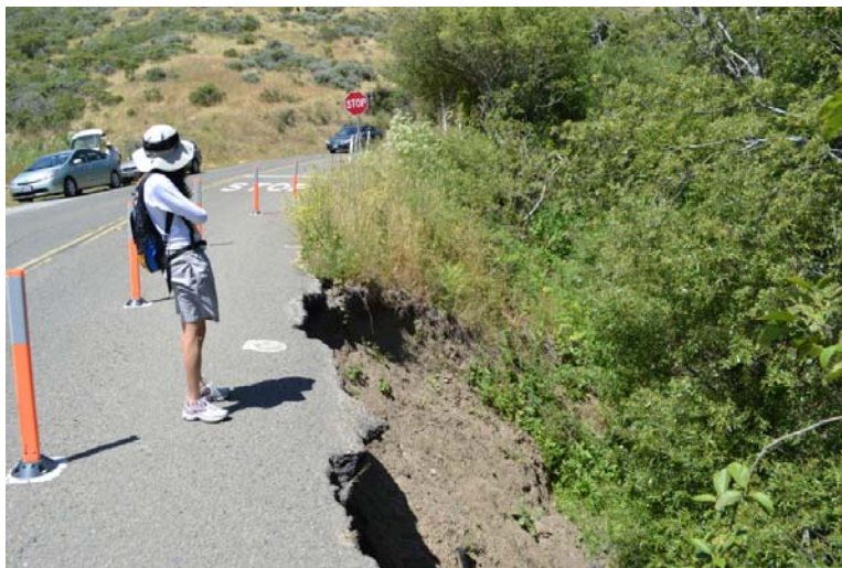
Failure of Muir Woods Road due to streambank erosion
