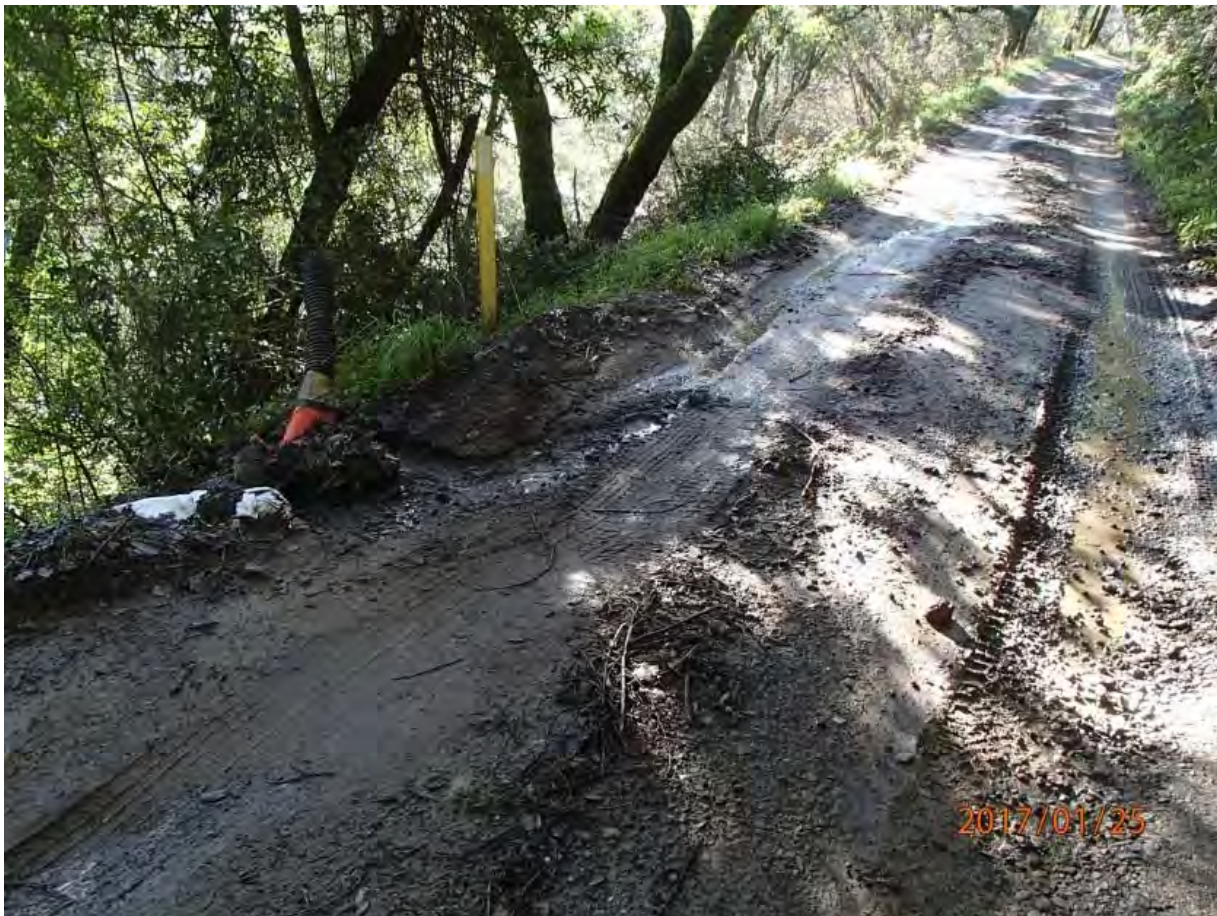
Photo 44. Photo taken of road surface discharge point Site #181. 700' of concentrated road runoff exits road at a low point in the road. Concentrated road run off has eroded a gully that delivers to Class II stream channel below.
