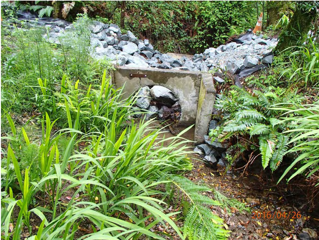
Photo 40. Photo taken looking downstream of failed and emergency repaired stream crossing at Site #204 at the remaining concrete headwall of the inlet and the installation of a temporary rock armored crossing.
