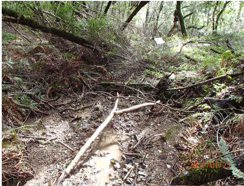
Photos 70 and 71. Photos of stream crossing Site #521.1. Culvert inlet is buried by sediment fan (left) and outlet of very undersized and poorly installed clay pipe is visible below the road (below).
