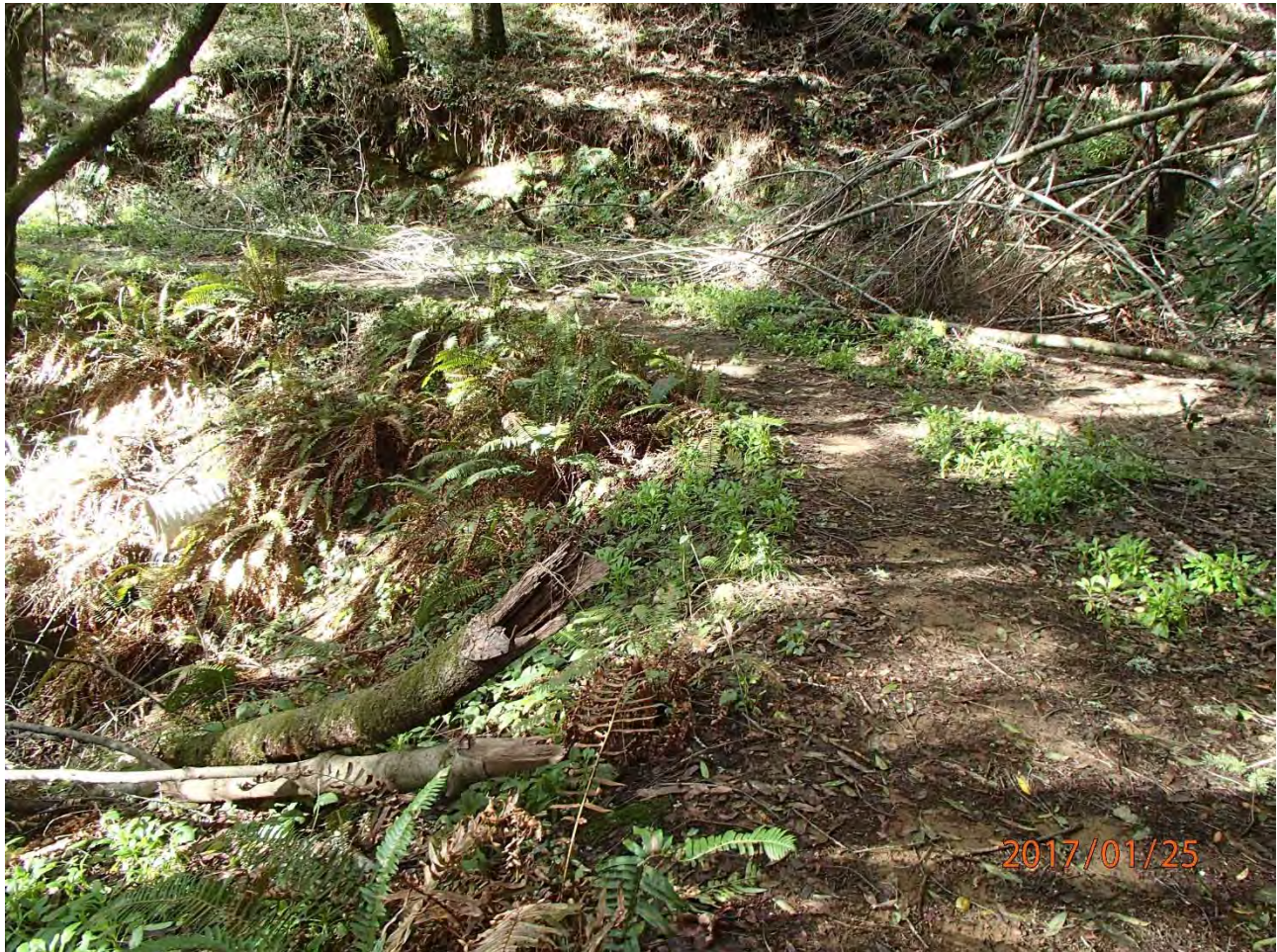
Photo 72. Photo of stream crossing site #522.1. Stream flow is being conveyed through a poorly installed, undersized and high plug potential 12" clay pipe at inlet and 18" aluminum pipe at outlet.
