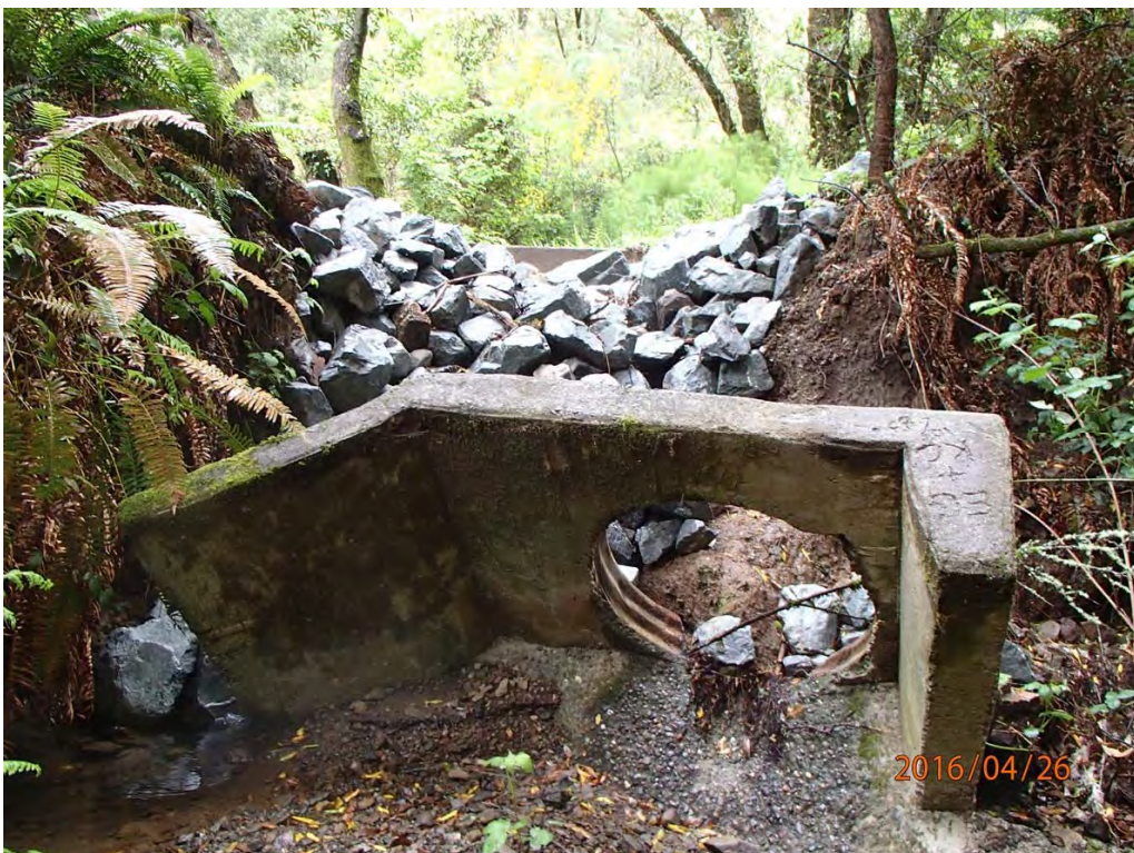
Photo 41. Photo taken looking upstream at failed and emergency repair at stream crossing Site #204 looking at the remaining concrete headwall at the outlet and the installation of a temporary rock armored crossing.
