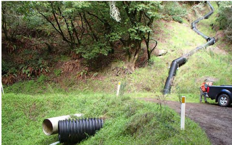
Photos 51 and 52. Photos taken of stream crossing Site #185. A rowdy Class 2 stream is conveyed through this crossing via an undersized 36" diameter HDPE plastic culvert with an aluminum flared inlet (left). There is a 24" diameter CMP ~26' to the right of the stream crossing that conveys flow from a failing downspout network upslope (right).
