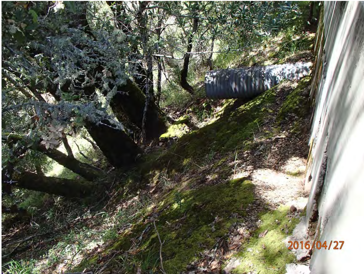
Photo 23. Photo taken from the outboard edge of the road looking downslope at the DRC outlet at Site #139. We recommend installing a downspout to the culvert outlet to protect the fillslope from future erosion.
