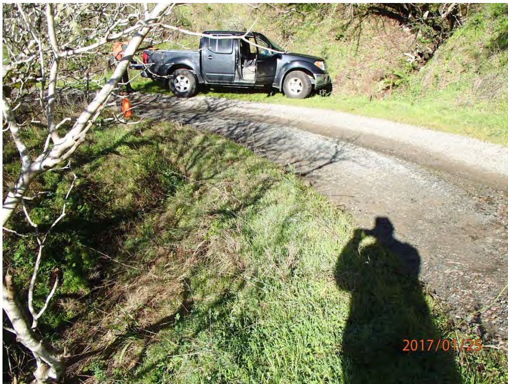
Photo 43. Photo taken of stream crossing Site #180. An undersized, 12" culvert is currently 100% plugged and not conveying flow through the pipe but underneath and through the fill. The site also receives significant runoff from the connected road reaches as well as Panoramic Rd. and Dipsea Trail above.
