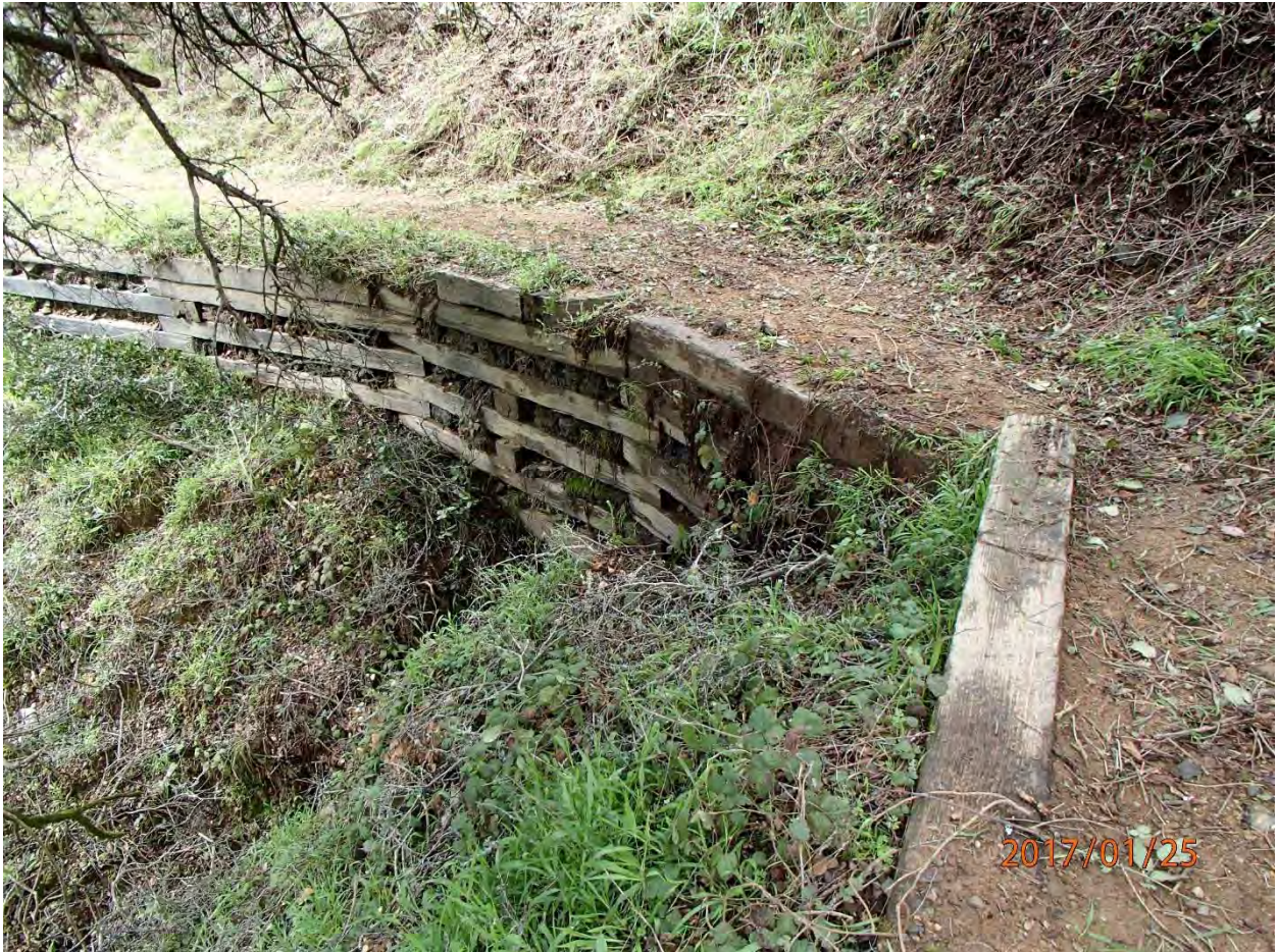
Photo 69. Photo of stream crossing Site #520. This near origin class 3 stream needs a properly sized and installed armored fill.
