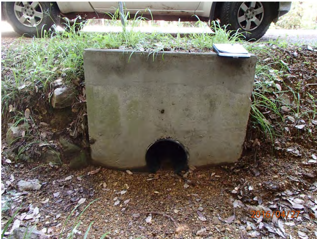
Photo 20. Photo taken from above the inlet of stream crossing Site #129. Note that the pipe has been recently upgraded with an 18” diameter culvert and 57” wide x 43” high concrete headwall. This site will require ongoing maintenance.
