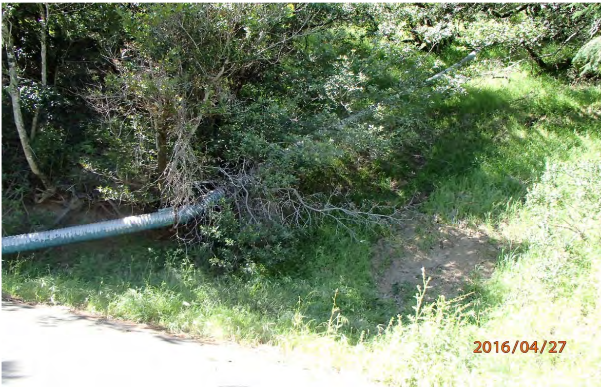
Photo 18. Photo taken of DRC Site #119 view of recently installed full round downspout attached to outlet to protect the fillslopes from further gullyng.
