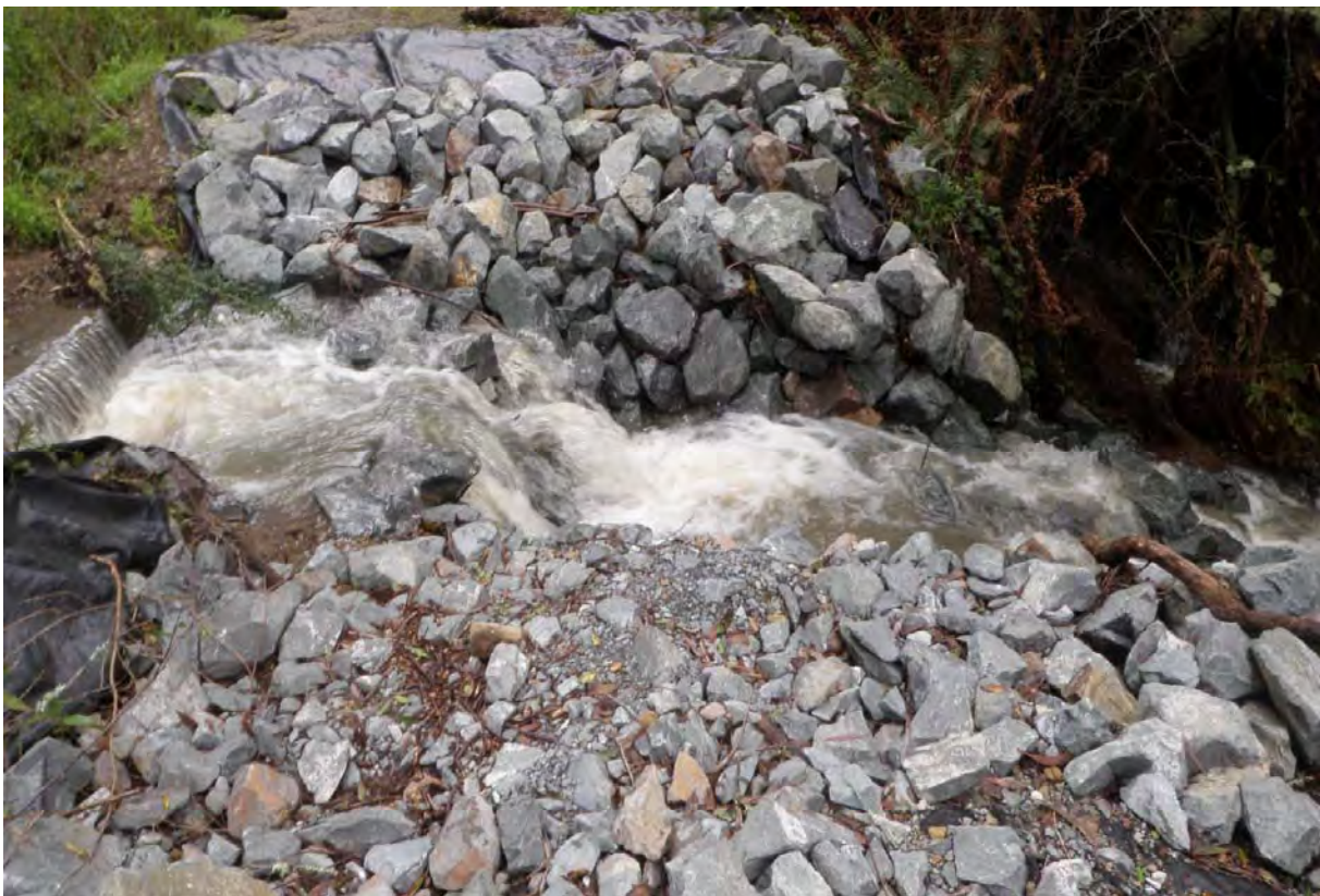
Photo 39. Photo taken from the right road approach in 2017 of failed stream crossing with subsequent adequate emergency repaired measures installed at Site #204.
