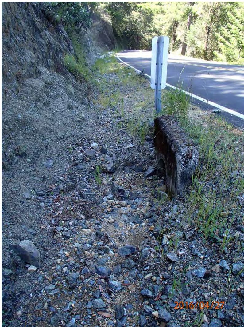
Photo 26. Photo taken along the inboard ditch looking down road at the inlet of DRC Site #143.
