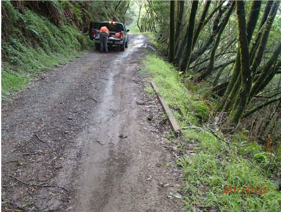
Photos 53 and 54. Photos taken of road surface discharge point Site #186. The concentrated RSDP run off is actively eroding a gully that delivers to Class 2 stream 100' downslope.
