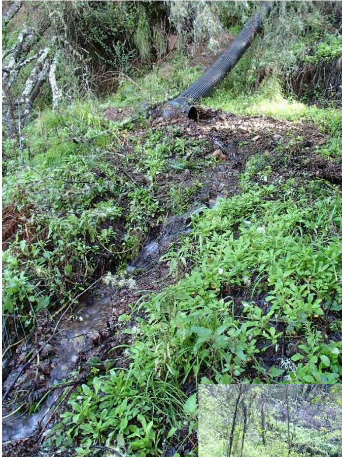
Photos 57 and 58. Photos taken of stream crossing Site #187.1. Stream flow from site #187 on Camino Canyon Road outlets onto this relict road prism (left). Stream flow is actively eroding through the fill and delivering sediment to the Class 2 stream downslope (below).
