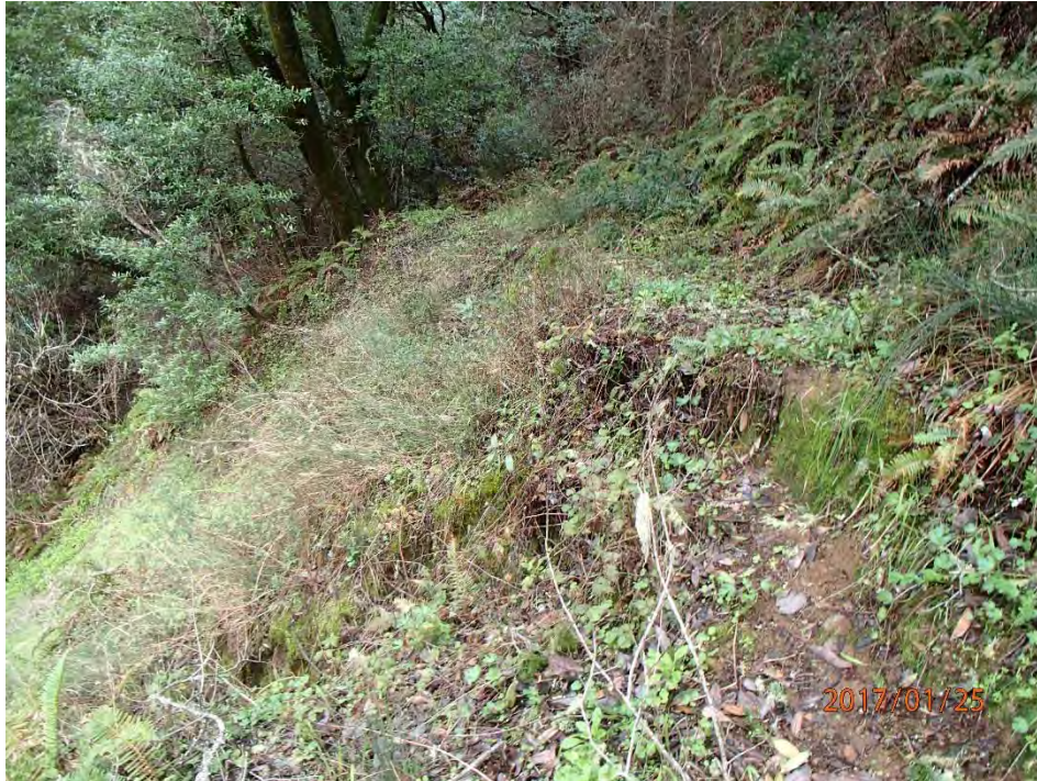
Photos 65 and 66. Photos taken of landslide Site #193. The road was decommissioned by NPS in 2003 when remaining perched fill was excavated. Currently, road and feature appear to be stable.
