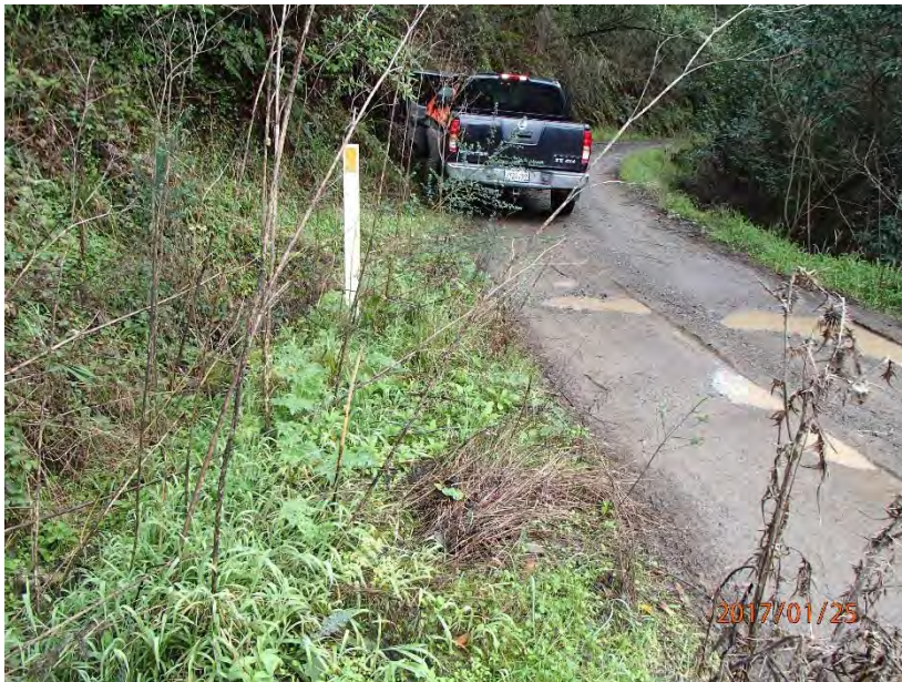
Photos 61 and 62. Photos taken of road beneath landslide Site #189. A large debris slide has deposited into channel below stream crossing site #188. Since failure, road has been rebuilt thru deposit with a maintained inboard ditch and DRC draining hillslope and feature seepage as well as road surface runoff.
