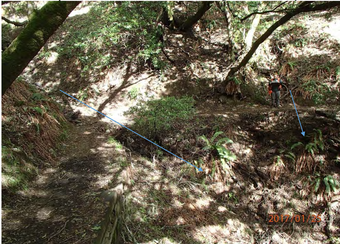
Photo 68. Photo taken of poorly installed and inadequately sized armored fill stream crossings at Site #517 (left) and Site #518 (right). Note the two blue arrows indicating flow at each crossing.
