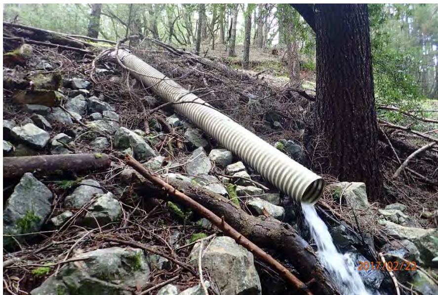
Photos 28 and 29. Photos taken of stream crossing Site #154. The small class 3 stream is conveyed through an 18" diameter culvert with an open inlet (top) and outlet with downspout onto an armored fillslope (bottom). Existing pipe is functioning well as installed. But, hydrologically connected road needs to be addressed with improved road drainage.
