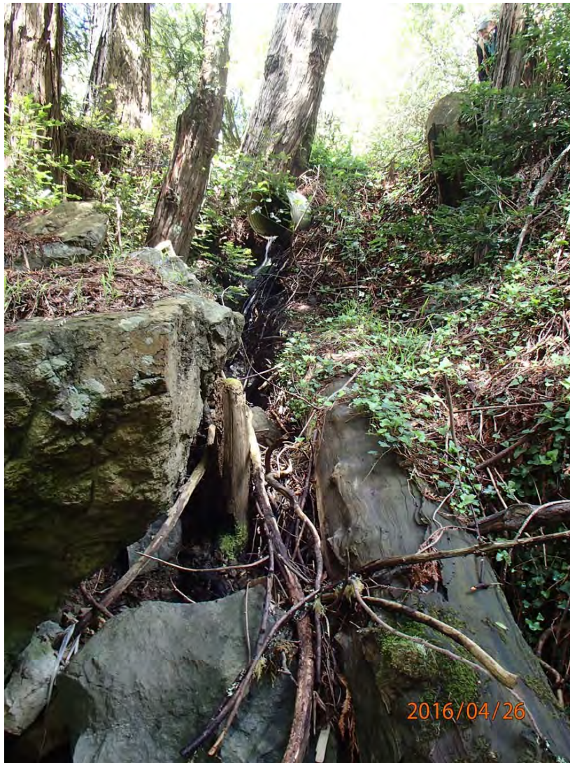
Photo 1. Photo taken from the trail looking upslope at the outlet of Site #78. We recommend installing a full round downspout to connect the outlet of this DRC to the armored trail crossing.
