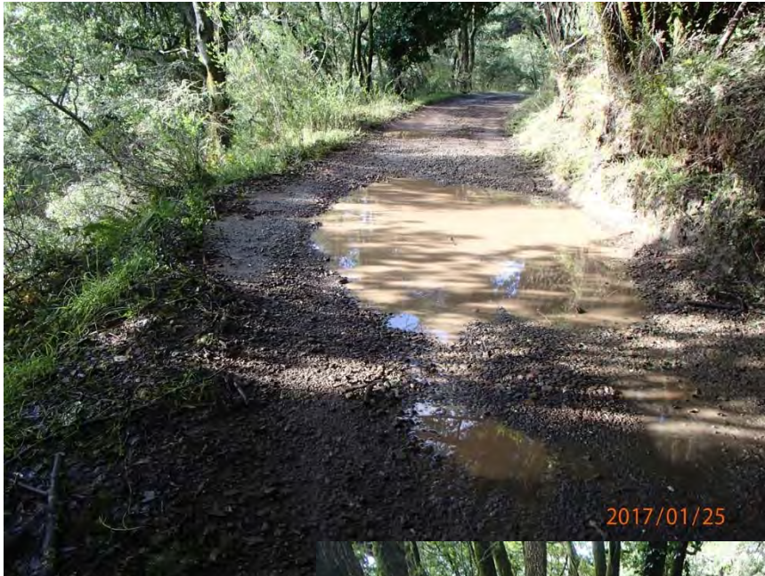
Photos 47 and 48. Photos taken of road surface discharge point Site #183. A section of insloped and bermed road accumulates water at 2 low spots 165' apart. At both sites ponded water exits road at OBF and is actively gullying the OBF slope.
