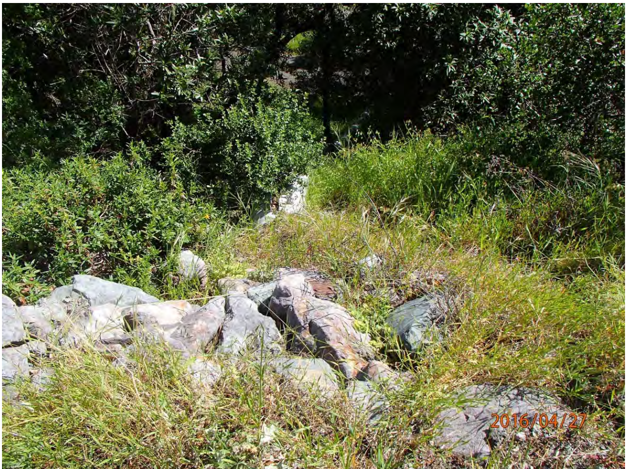
Photo 27. Photo taken of the armored outlet at stream crossing Site #152. The culvert is undersized, but at time of re-evaluation, the inlet was open and the pre-existing sediment fan above inlet had been cleared.
