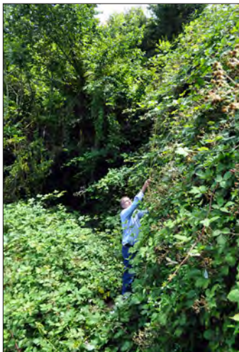
Figure 3.8. Invasive blackberries to be removed along the East Black Point slope walk and retaining wall between Quarters 2 and 3. View looking south, 2011 (OCLP).
