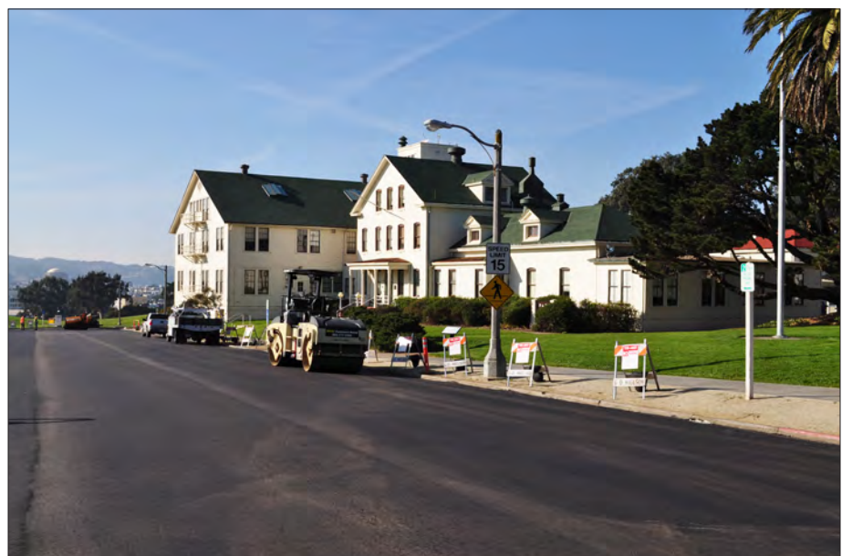
Figure 3.52. Parking area along MacArthur Avenue to be made accessible with new parking spaces, compliant curb ramps, and a refurbished planting strip. View looking west, 2011 (OCLP).
