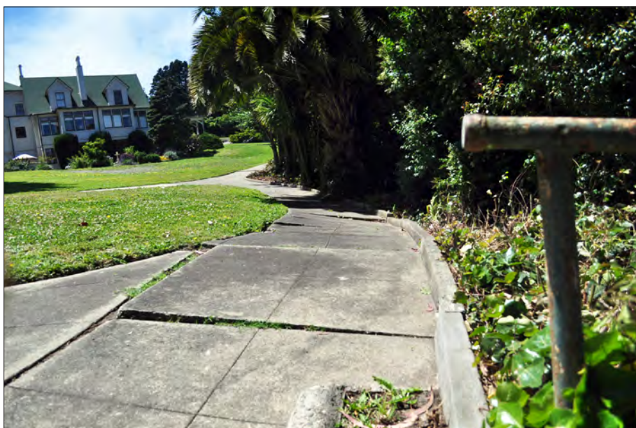
Figure 3.12. Heaved and cracked concrete walks at the crest of the East Black Point slope to be replaced in-kind to accommodate safe public access. View looking north, 2011 (OCLP).
