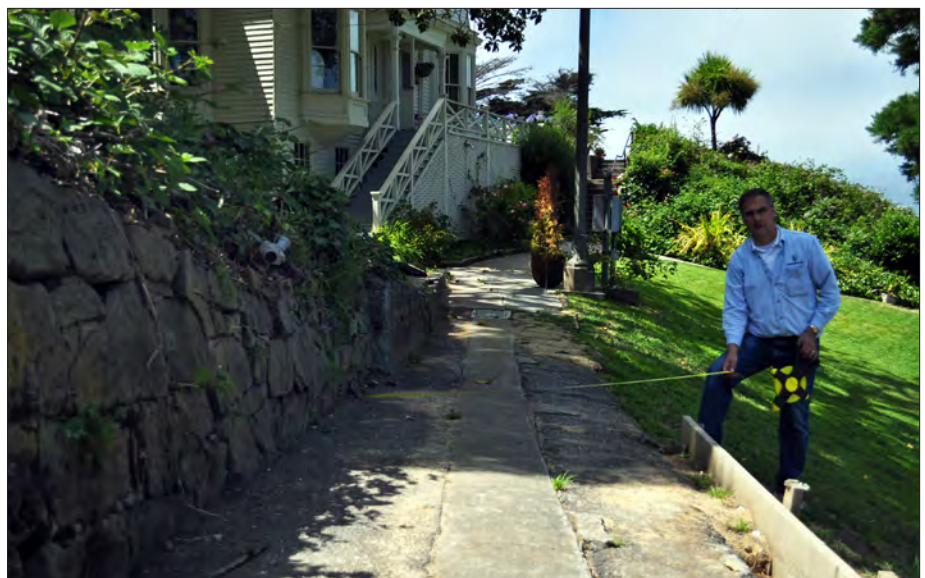
Figure 3.20. Deteriorated concrete walk adjacent to Quarters 4 to be leveled and replaced in-kind. View looking north, 2011 (OCLP).
