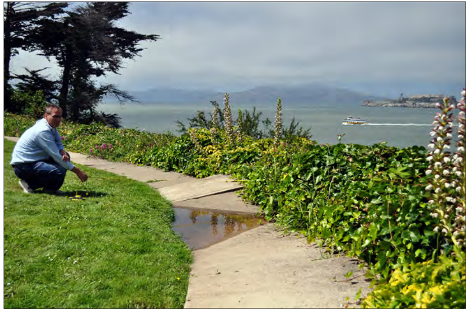
Figure 3.41. Concrete walks on the Quarters 4 garden terrace to be removed and replaced in-kind to remedy undulations and standing water due to poor sub-surface drainage and seismic activity. View looking north, 2011 (OCLP).
