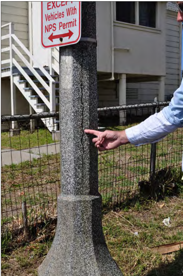
Figure 2.7. Cracked cast-concrete pole light to the west of Building 231. View looking southeast, 2011 (OCLP).
