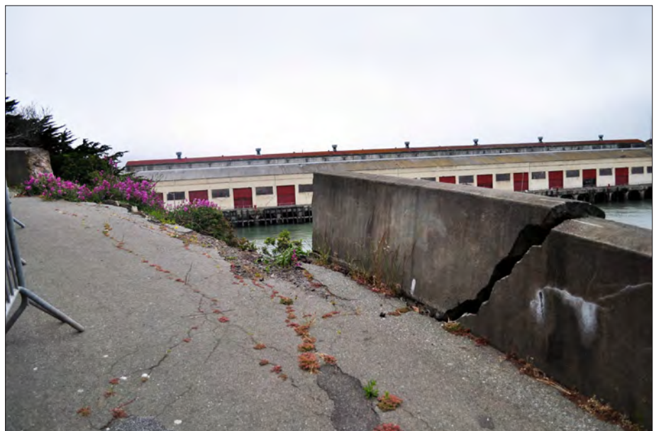
Figure 3.42. Collapsed concrete retaining wall along McDowell Avenue to be replaced consistent with road narrowing to enhance visitor safety. View looking west, 2011 (OCLP).
