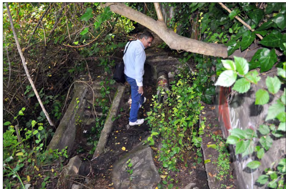
Figure 3.11. Collapsed concrete walks and drainage structures on the East Black Point slope to be rehabilitated to support visitor use. View looking south, 2011 (OCLP).
