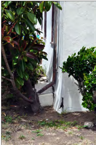
Figure 3.115. Positive drainage away from the Quad buildings is to be provided to prevent further facade damage, shown here at Building 38. View looking north, 2011 (OCLP).
