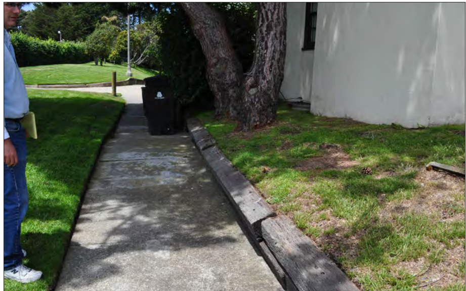
Figure 3.23. Timber wall along west side of Quarters 7 to be reset. View looking north, 2011 (OCLP).
