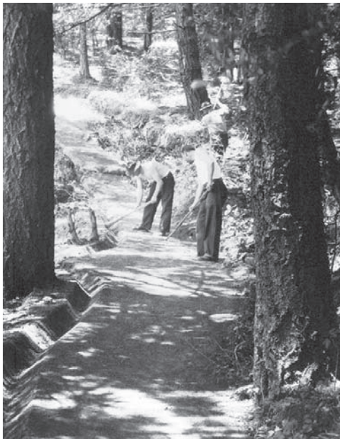
Figure 4.42: CCC/CWA crews at work on the Dipsea Trail through the northwestern corner of Muir Woods, June 1934. Note drainage swale along left side of trail. J. Barton Herschler, Muir Woods June 1934 monthly report. National Archives II, College Park, Maryland, RG 79, PI 166, E7, Central Classified Files, 1933-1949, Muir Woods, box 2293.
