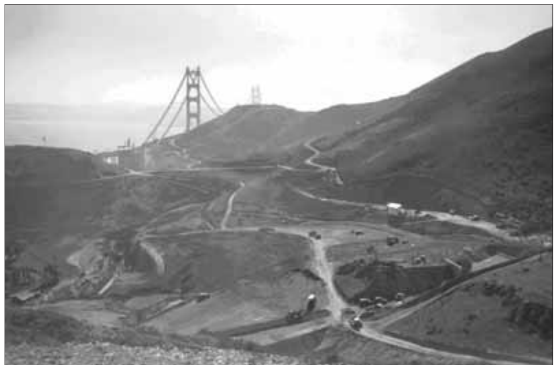
VG11 Construction of Highway 101 and Alexander Avenue resulted in the creation of extensive cut and fill slopes. The resulting revegetation efforts may have introduced invasive plant species to the open areas of Fort Baker. Date: November 9, 1936 (Golden Gate Bridge Archives).
