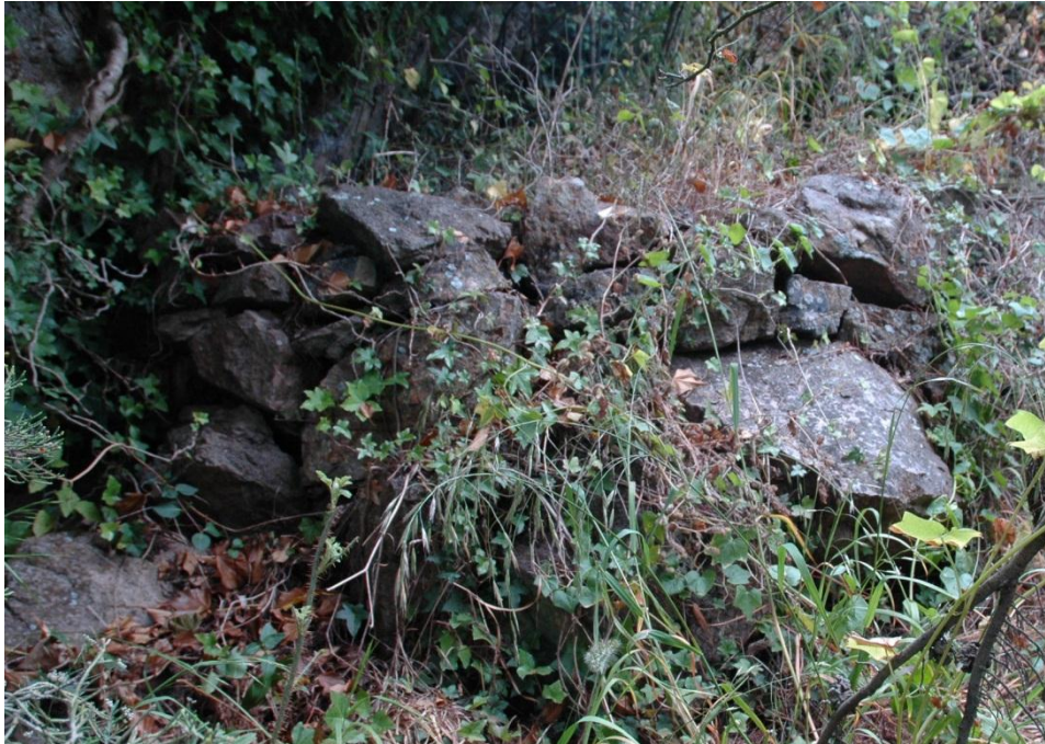
Detail of one the garden terrace stone walls, located east of the Main House.
