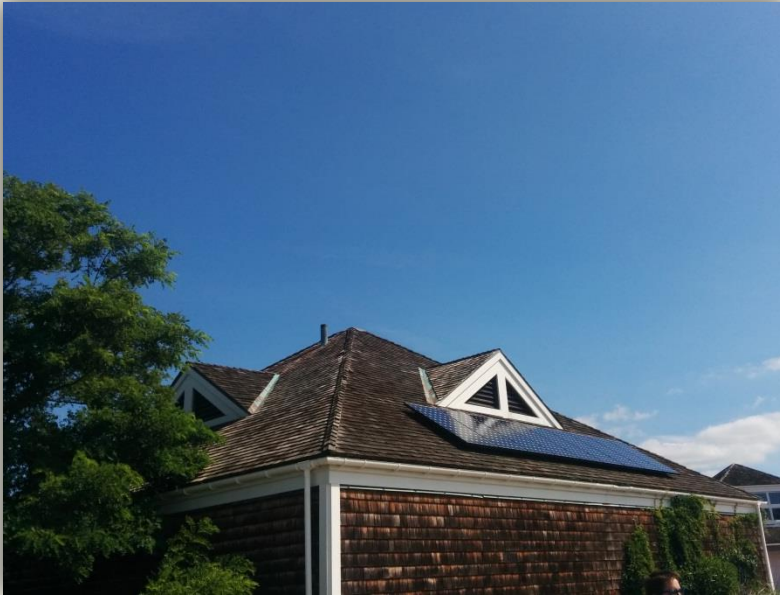
Grid Tied Solar Panels at North Shore Observation Deck
