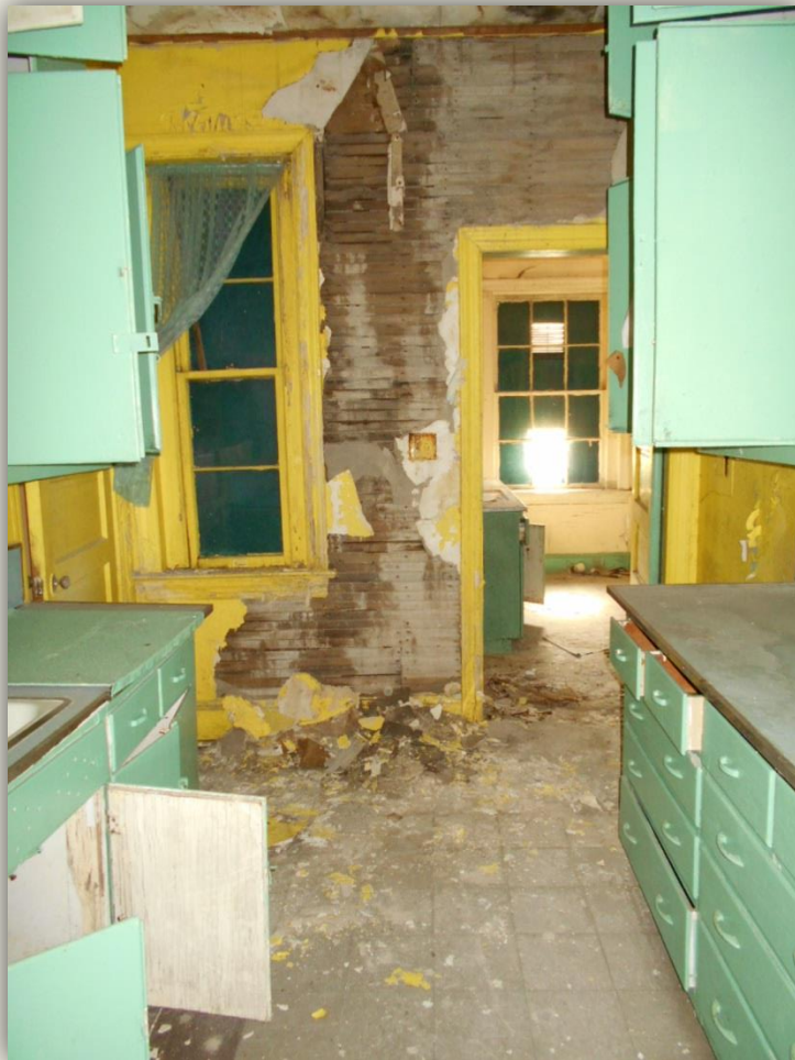
Potentially Hazardous/Toxic Materials in Building 7 Kitchen
