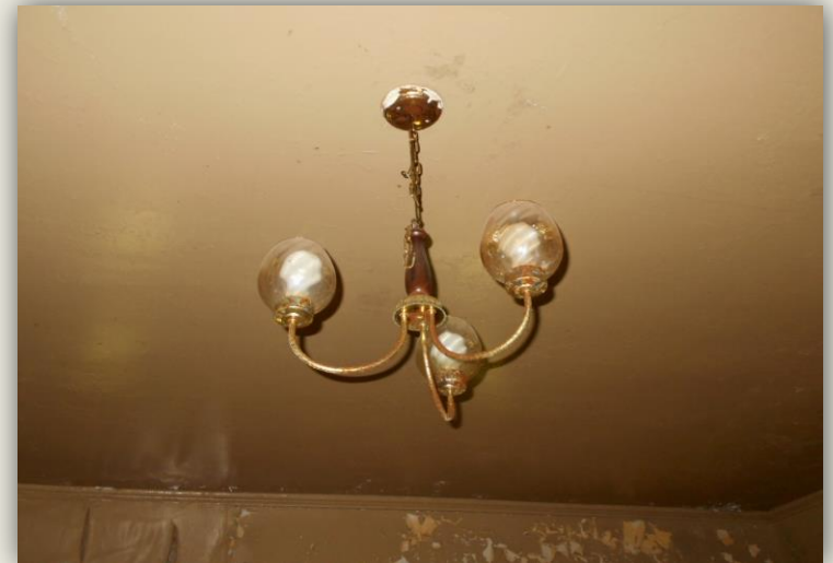
Existing Light Fixture in Bldg. 7
