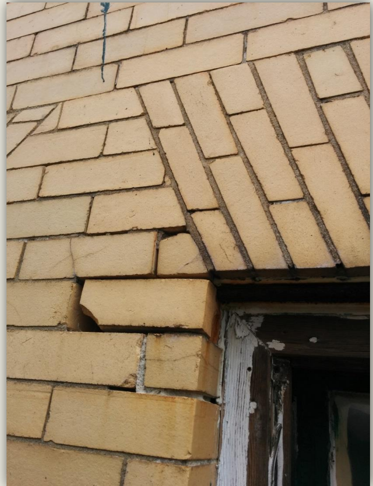
Building 7 Exterior - Loose Bricks Around Window
