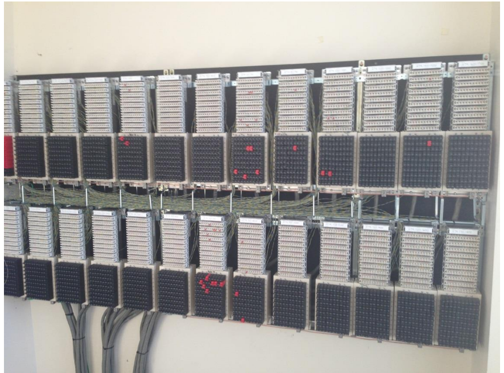
Verizon rebuilt frame in B26 (2013)
