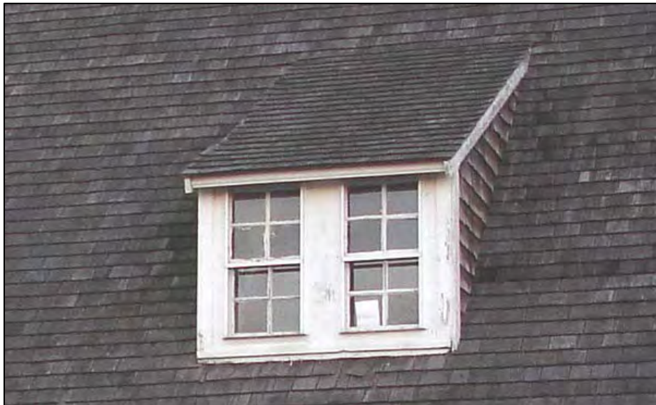
Figure 48. Spermaceti Cove Life-Saving Station, west elevation dormer window openings (W207 and W208).
