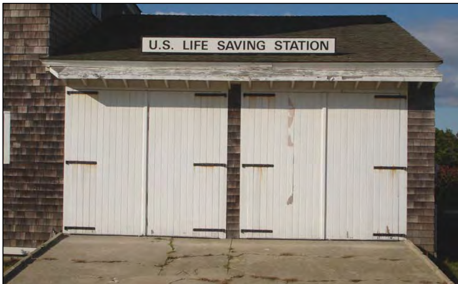
Figure 46. Spermaceti Cove Life-Saving Station, east elevation Boat Room doorways (D105 and D106).
