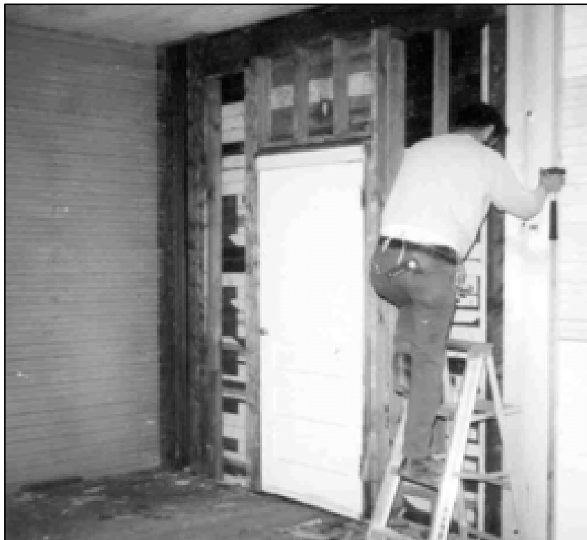
Figure 37. Spermaceti Cove Life-Saving Station, Feb/March 1975 depicting interior of Boat Room north wall enclosing wide doorway.
