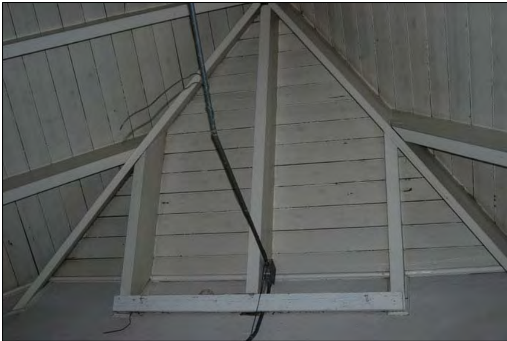
Figure 60. Spermaceti Cove Life-Saving Station, Room 206 interior view of clipped-gable roof framing looking south.
