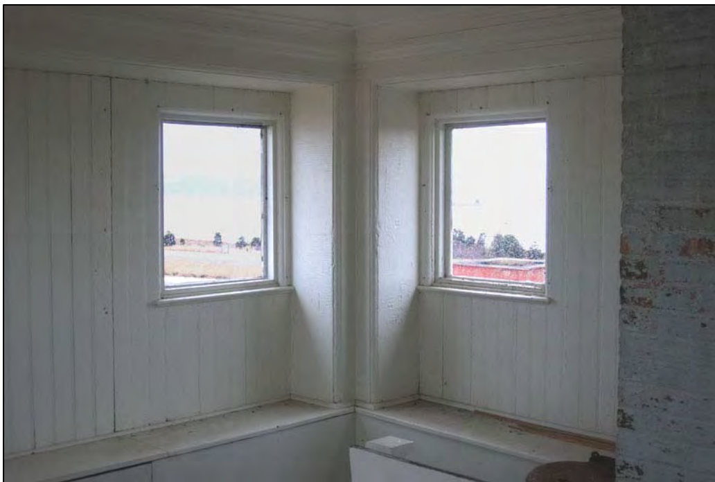
Figure 64. Spermaceti Cove Life-Saving Station, Watch Room/Room 401 looking southwest depicting cantilevered window section and typical woodwork for the fourth story.
