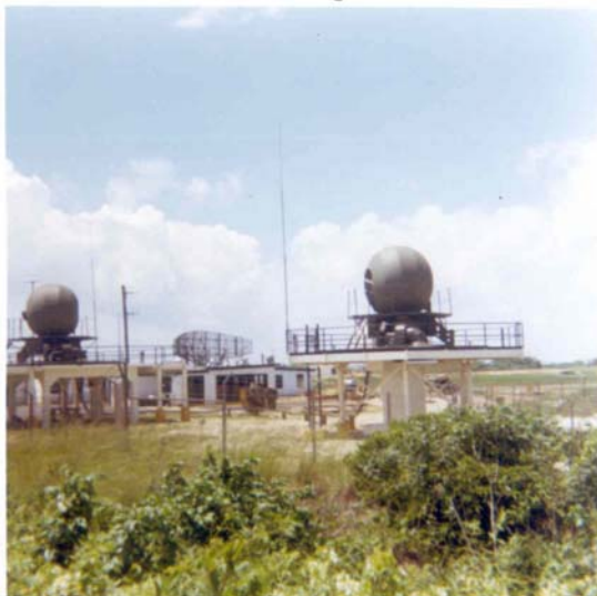
Image of the Nike radar equipment at Fort Hancock. Ronald Kacsmar serviced these and others on site while employed with the U.S. Army Ordnance Department.
