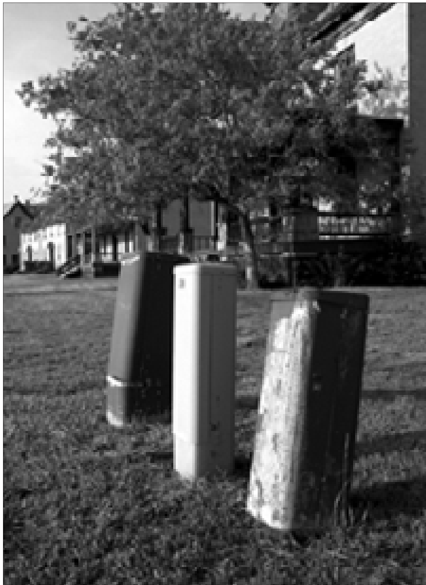
Figure 2.4. Above ground utility boxes are located throughout the study area, notably between the buildings of Officers Row, as pictured above. These fixtures should be located to one side of the gap between Officers Row quarters or underground, rather than in the center of the open space. OCLP, 2004.
