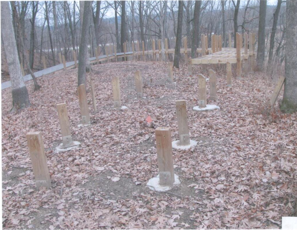
Figure 4. Detail of boardwalk construction showing posts set in concrete on surface of mound (NPS-MWAC photo).
