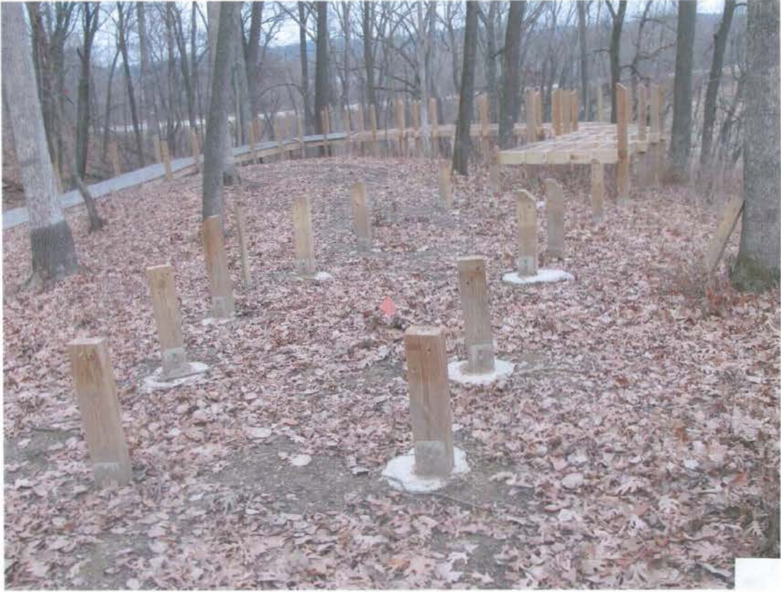
Figure . Detail of boardwalk construction showing posts set in concrete on surface of mound (NPS-MWAC photo).
