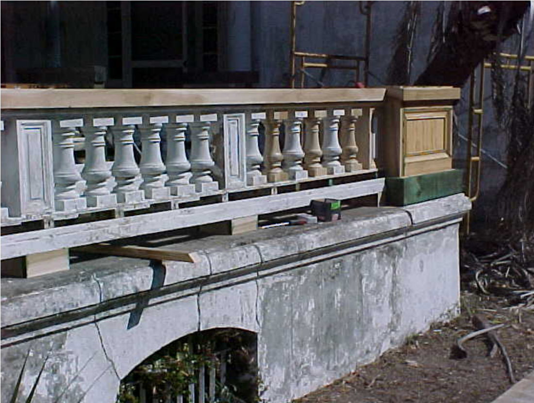
Wood stabilizer applied as a primer to unpainted wood repairs just prior to painting. Plum Orchard Mansion, Cumberland Island National Seashore.
