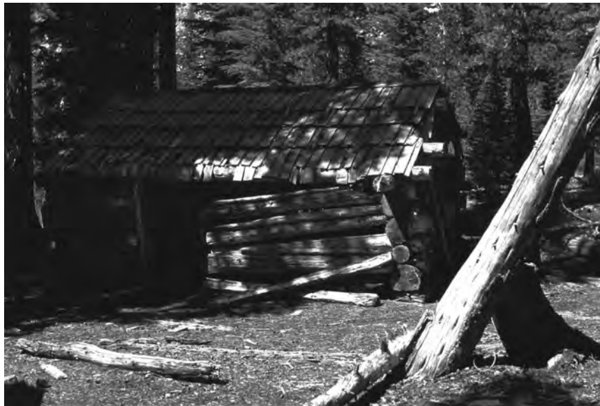
1981 photo of a partially collapsed structure at the Minaret Mine site. (Devils Postpile National Monument image collection)
