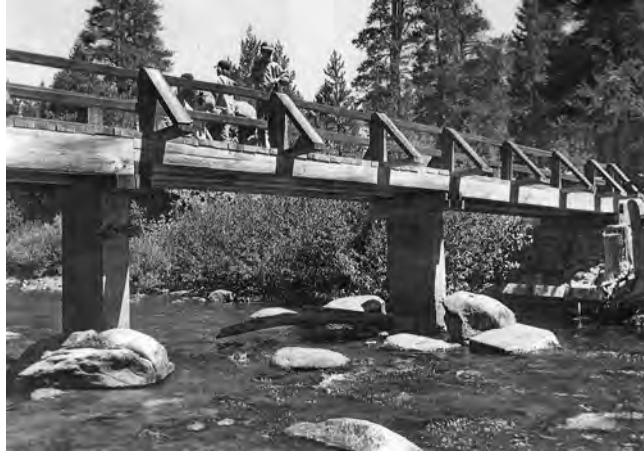
Postpile–Soda Springs Meadow Bridge. Note the cracked piling on the left, 1970s. (Devils Postpile National Monument image collection)
