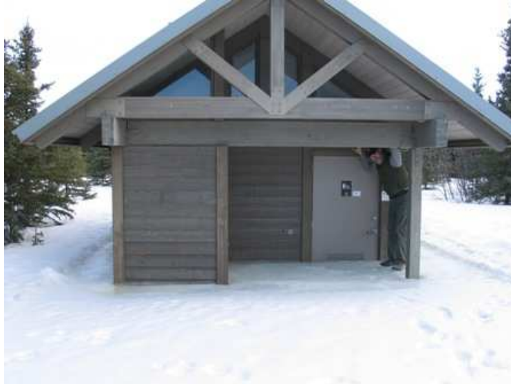
Restroom in Teklanika River Campground inundated by ice overflow (West District Roads Supervisor Brad Ebel standing on ice to right of bathroom door)
