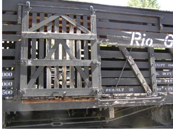
Figure 109. Rotten door sill
