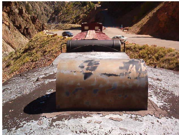
Figure 83. Roof top of engineer cab in bad condition
