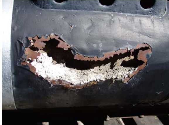
Figure 64. Corrosion has left a growing hole in the steam piston barrel
