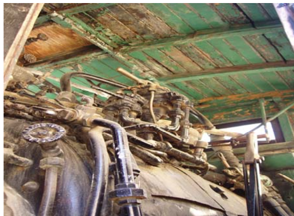
Figure 66. Engine room ceiling, peeling paint and rotting wood
