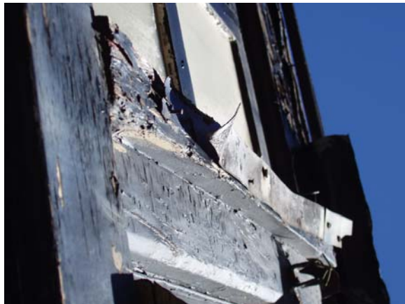
Figure 73. bent metal part on window of engineer cab
