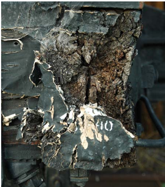
Figure 108. Right side A end rotten end beam
