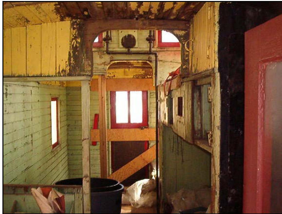
Figure 104. Deterioration and neglect found in the Caboose. Notice the roof rot and the left side is missing most of its interior integrity.
