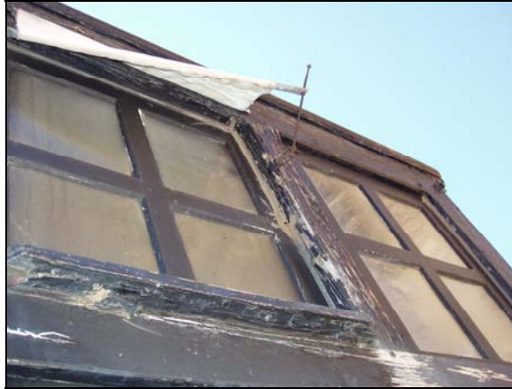
Figure 75. Peeling paint and rotten wood on engineer's cab
