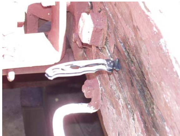
Figure 90. Rotten A end beam
