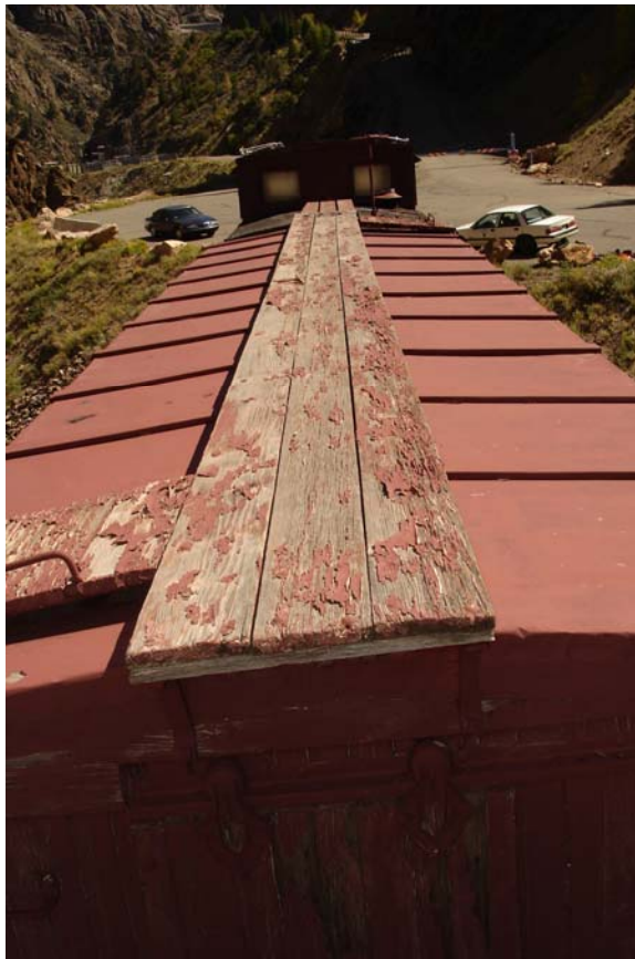
Figure 95. Paint on roofwalk is peeling
