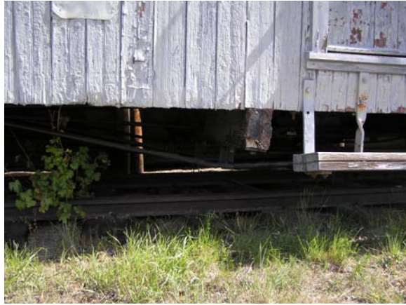
Figure 124. Rotten wooden beam
