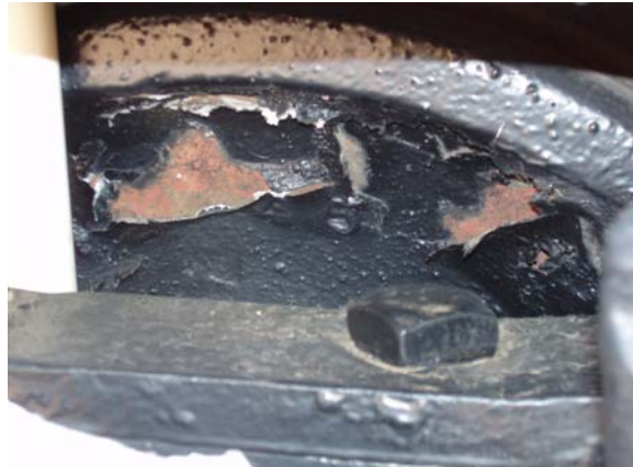
Figure 65. Peeling paint and rust materials
