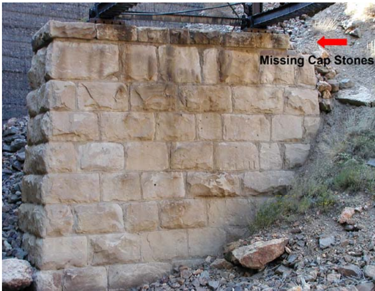
Figure 134. Piers are overall good condition, however, two missing cap stones are found on west pier
