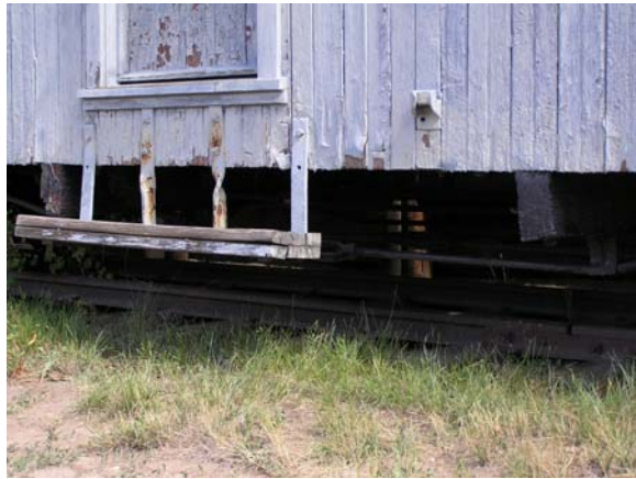
Figure 123. Deteriorated foot board on the side
