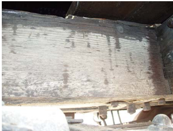
Figure 79. Weathered wood frame
