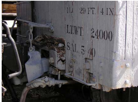
Figure 120. Rotten wooden part around coupler pocket of B end
