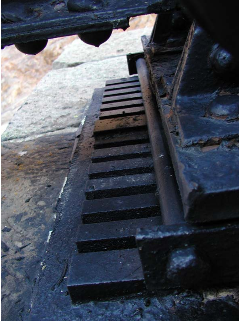
Figure 137. Roller bearings are frozen due to lack of movement
