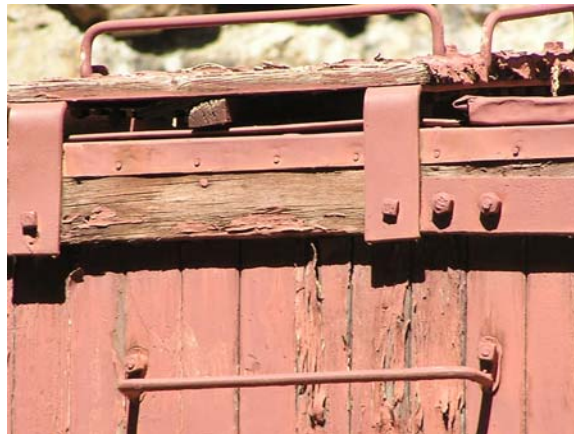
Figure 87. Fascia is rotten and needs to be either repaired or replaced with in-kind materials
