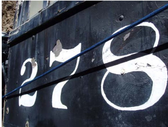
Figure 78. Paint peeling on side letters
