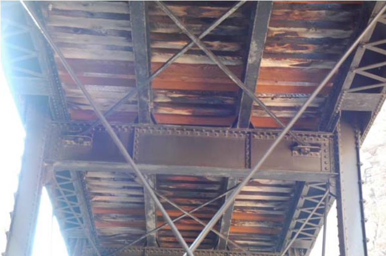
Figure 130. Ties damaged by water and rotten metal parts
