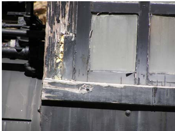
Figure 74. Weathered window frame
