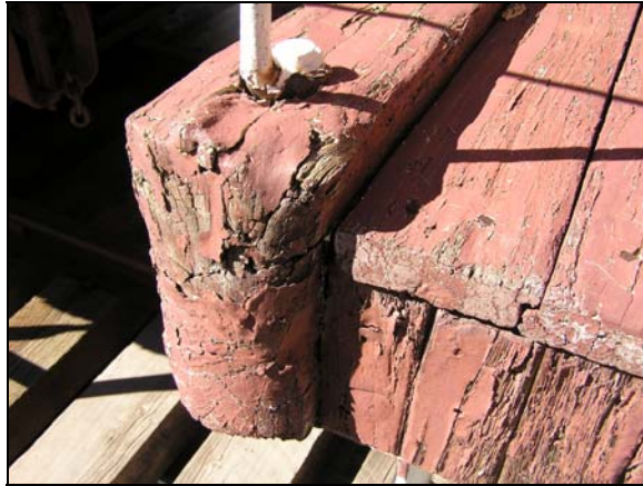
Figure 100. Wood Rot and paint peeling on the A end deck and end beam
