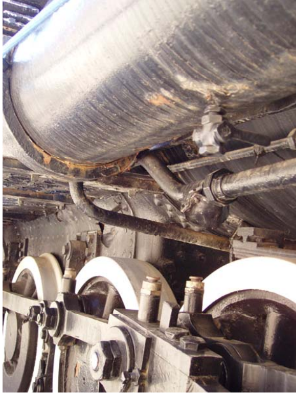
Figure 80. Rust under smoke box
