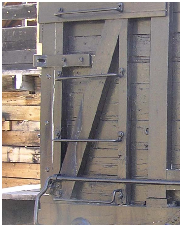
Figure 116. Vertical crack on the post of A end
