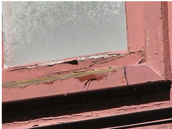
Figure 103. Paint peeling on windows and window sash
