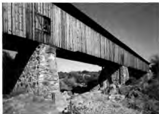
The Knights Ferry Bridge in Stanislaus County, California, shown here in this 2004 photograph, dates from 1864. (Photograph by Jet Lowe, courtesy of the National Park Service)
