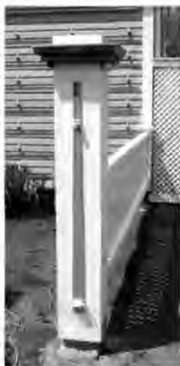
FIGURE 3 This view shows the repairs made to the gate posts. (Courtesy of Longfellow National Historic Site)
