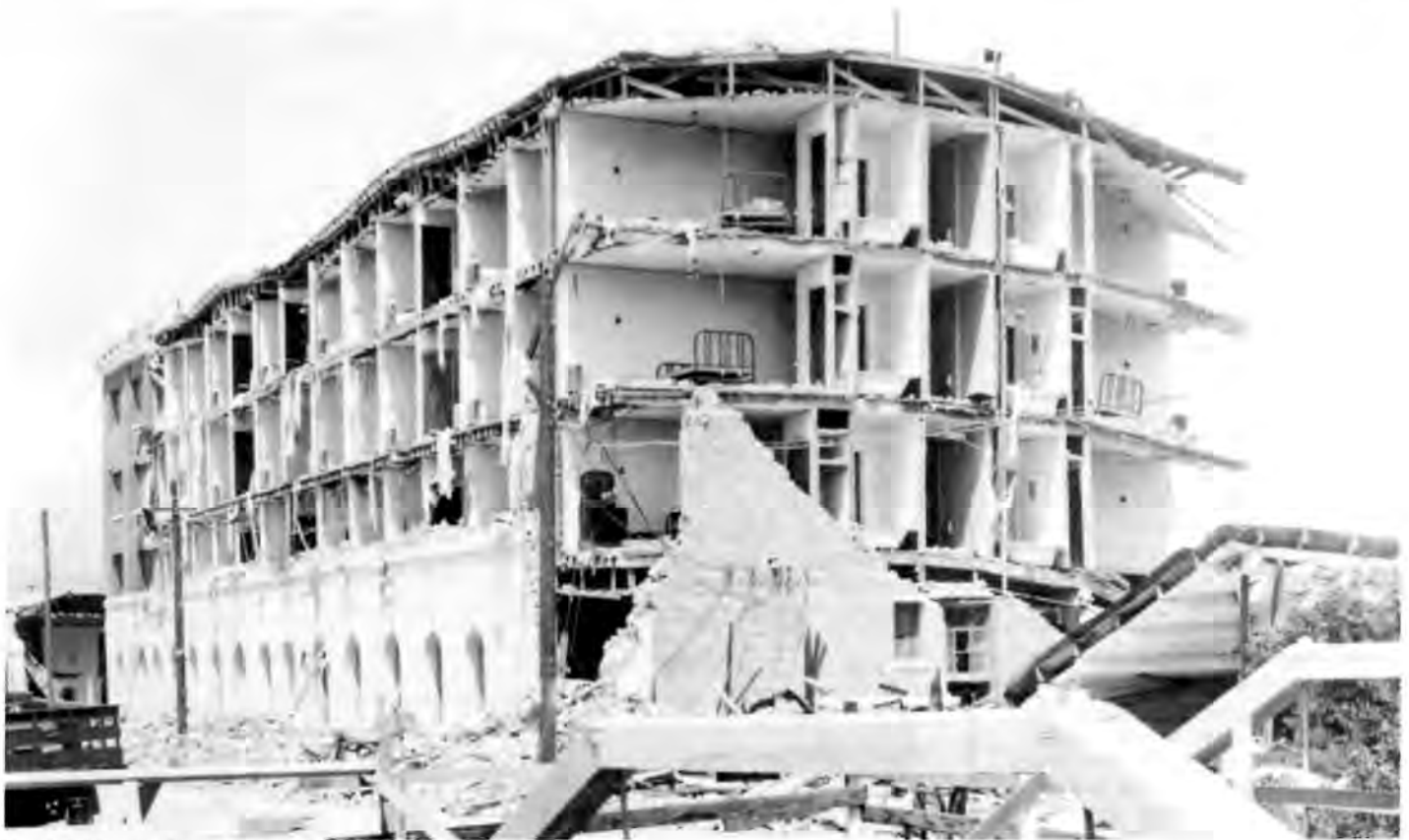
Hotel California after 1925 Santa Barbara Earthquake.
