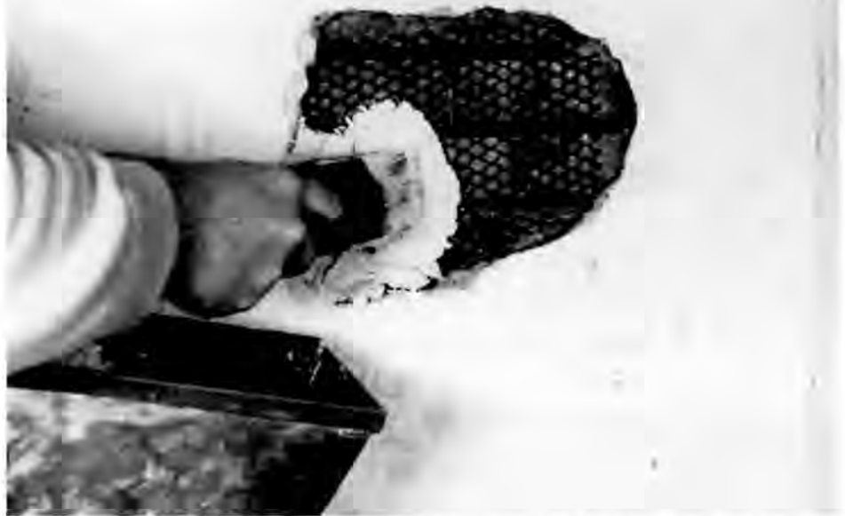
The wood lath has been covered with a small piece of diamond mesh lath (attached to the wood lath with a tie-wire). The plasterer will apply one or two ready-mix gypsum basecoats. After they dry, the gauged lime finish coat will be applied. Photo: Walter Jowers.
