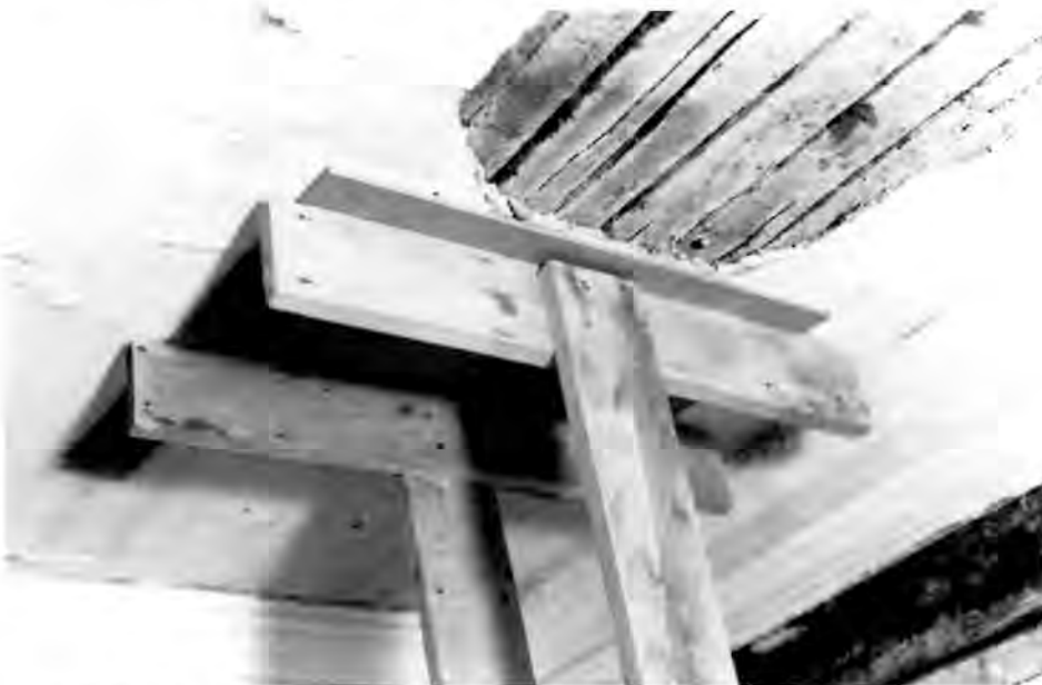
After applying an adhesive to reattach sagging ceiling plaster to the wood lath, a brace is used until bonding is complete. Photo: John Leeke
