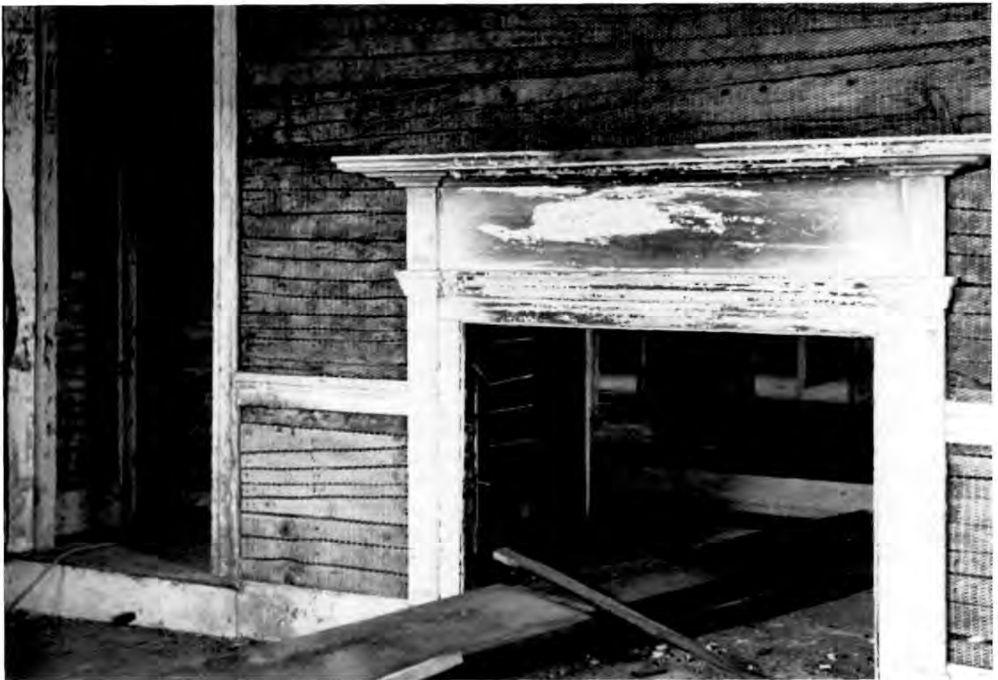
In this project, the split-board lath has been covered with diamond mesh lath in preparation for new coats of plaster. This method permits the early lath to be saved while the metal lath, with its superior keying, serves as reinforcement. Photo: National Park Service files.
