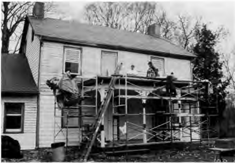
Park construction crew led by preservation carpenter Doug Townsend rehabilitates the covered porch. A new flat seam metal roof was installed with assistance from the NPS Historic Preservation Training Center in Frederick, MD. NPS photo.
