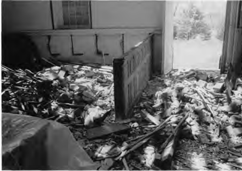
Twenty-two tons of brick, mortar, plaster, lath, and framing fell to the sanctuary floor crushing four box pews and two original deacon benches. The debris was carefully sifted for all salvageable materials. Photo taken May 23, 1996.
