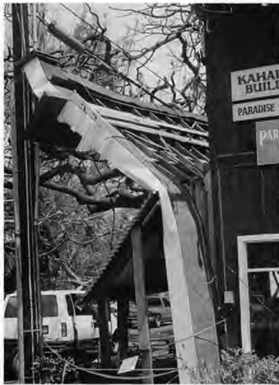
Hurricane Iniki in 1992 ripped the façade from this one-story vernacular store building on Kauia, Hawaii. The utility pole prevented the façade from falling onto the sidewalk and road. Photo courtesy David W. Look.
