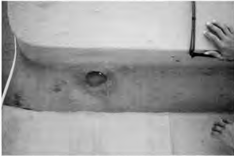
Painted many times, the corroded galvanized steel roof had many leaks. Here a gutter is cracked and leaking badly next to a critical rainwater outlet. The outlet was one half the size that it should have been. This causes overflowing and even worse leaks during tropical down-pours.
