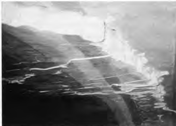
Large cracks in the vaults with relative movements of around 25 cm.
