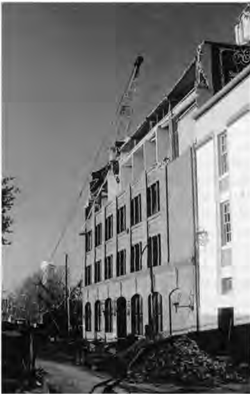
By progressive failure the unreinforced-brick parapet and fourth-floor façade of this building on Bluxome Street collapsed onto the sidewalk and street during the Loma Prieta earthquake killing six people in a car pool.
