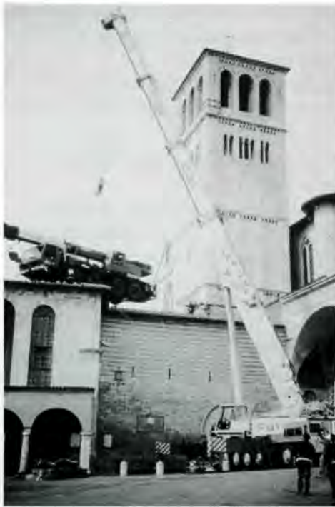
A crane in front of the convent lifts a second crane over the wall into the courtyard.
