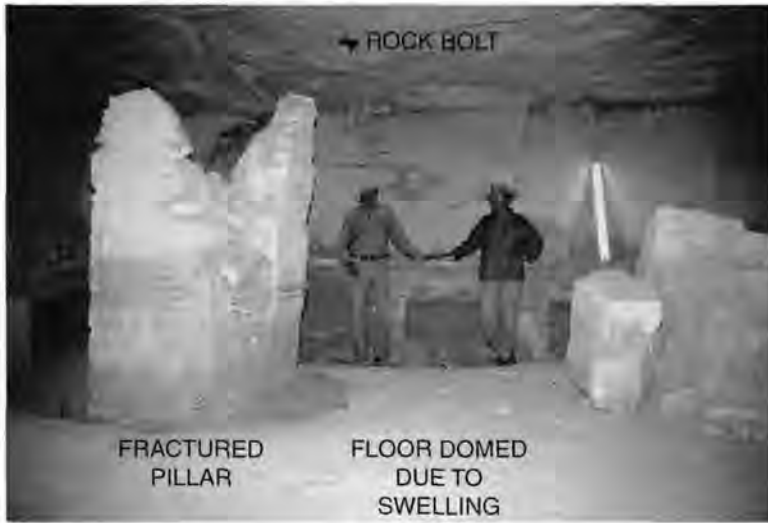
Interior view of a lower chamber in the tomb of Ramesses II, KV-7, an example of the damage caused by successive flood events. Virtually all of the decorative plaster reliefs are lost, and the rock structure has been heavily impacted by swelling of the underlying shale. The floor obscures the two team members' feet because it has swelled in the center. There are two rock pillars on either side that have fractured and collapsed. At the top is a rock bolt installed by another project in a recent effort to forestall further spalling of the ceiling. Photo by James McLane.
