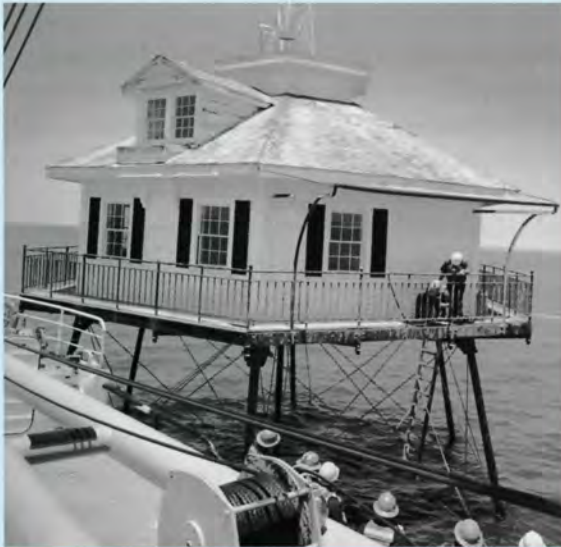
White Pine conducting maintenance work on midbay lighthouse in Mobile Bay. Crew is removing ladder from lighthouse for repairs. White Pine crane and winch are in foreground. To avoid getting in the way of a very active crew, this shot had to be taken without a tripod. Bright light enabled stopping down for depth of field while maintaining a relatively fast shutter speed.
