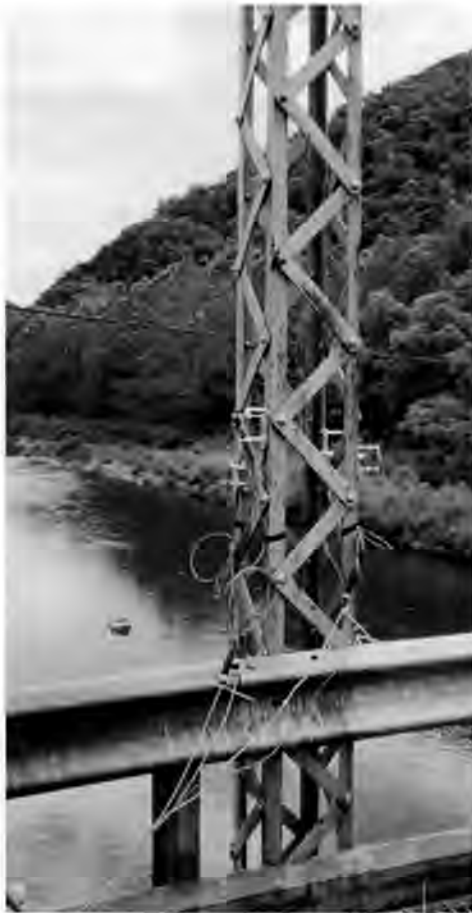
Detail of vertical member (labeled U11-L11 in drawing on next page), with strain gauges installed for load testing. Photo by author, 1998.
