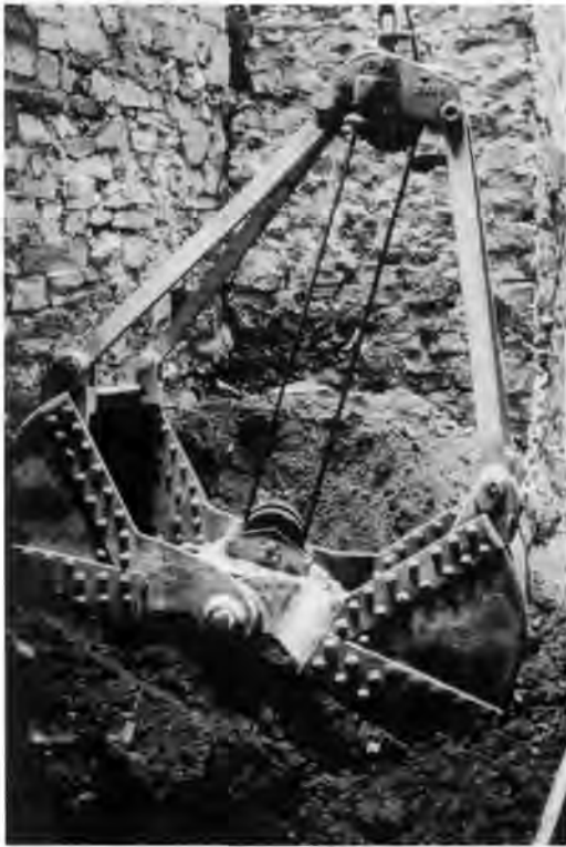
Monitoring excavations at the St. John's Bastion, Quebec City. Photo by Robert Gauvin.
