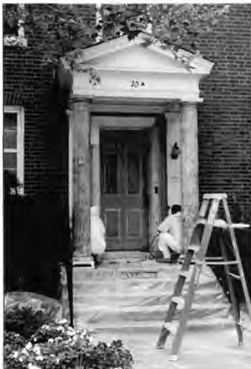
Quarters 20A at Fort Myer, Virginia. Repair of deteriorated wood at the front entrance, and complete paint removal and repainting. Photo by the author.
