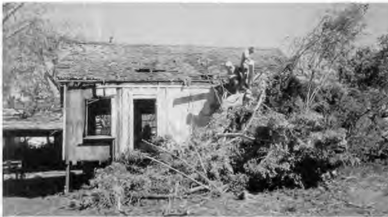
Bay View, Kalaupapa National Historical Park. National Park Service crew removing over-grown vegetation at the beginning of the rehabilitation project. Photo by Hunter Glidewell.
