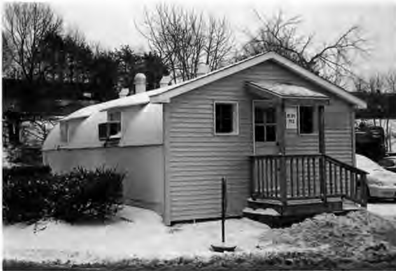
False fronts were often applied to Quonsets in order to create a more traditional look. Even the Navy, who converted this one into offices at the Subase in Groton, Connecticut, disguised the semi-circular Quonset form. Photo by the author.
