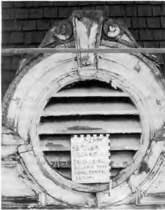
Bullseye showing lead paint failure. Below: Bullseye and parapet with new metal plate.
