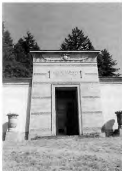
Distinctive features of the mausoleum, such as the precast concrete entrance pylon and flanking urns, the bronze doors, and the amber-colored glass windows, suffer from vandalism and a lack of maintenance.
