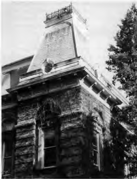
Southeast tower of Villard Hall before restoration. Photo by George Bleekman III.
