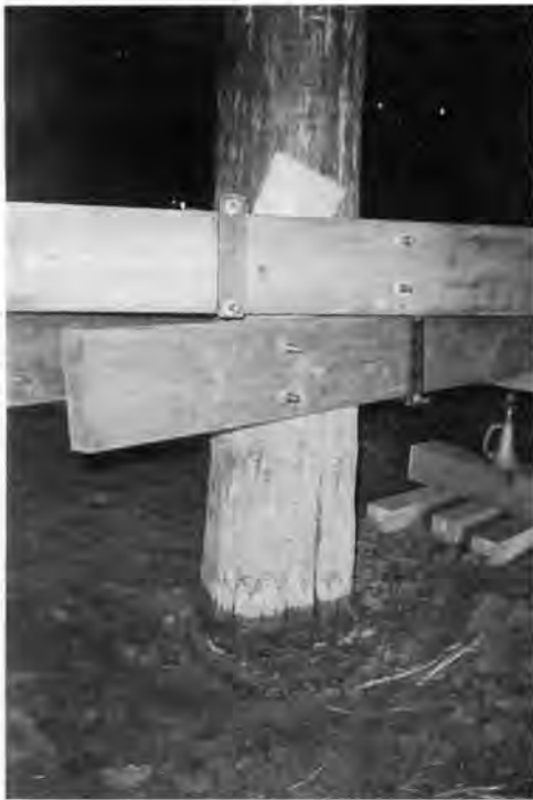
Temporary bracing supports an interior post while the concrete cures below it. Photo by David Pinyerd.
