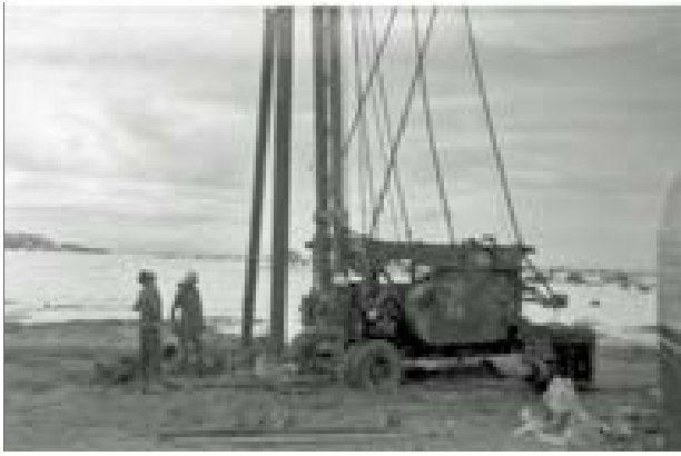
Well drilling, Willow Flat, Island in the Sky, January 1968. C 40911.171, SEUG Photographic Archives. The NPS could not find adequate water on the Island in the Sky mesa top, forcing the installation of large water tanks. This dynamic was repeated in the 1970s at Hans Flat, serving the Maze District.
