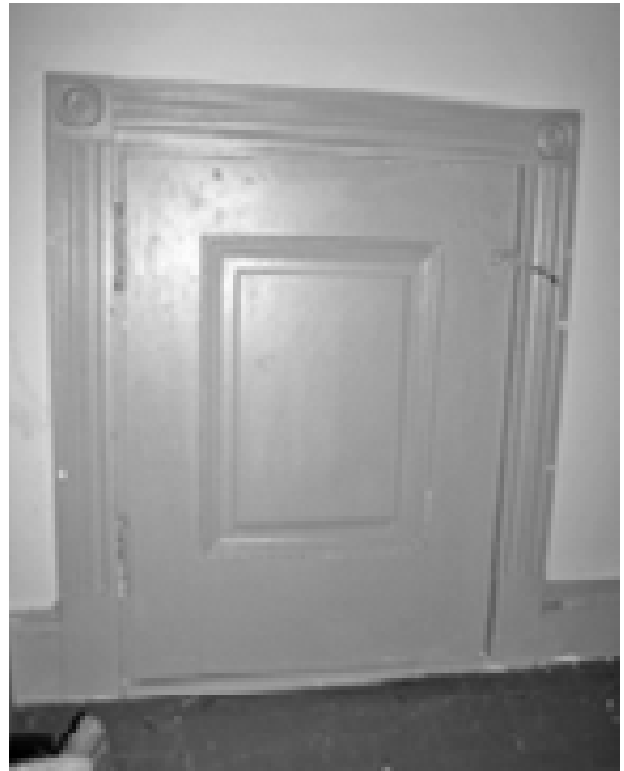
FIGURE 138. View of closet door in Room 202. (T. Jones, NPS, 2005)
