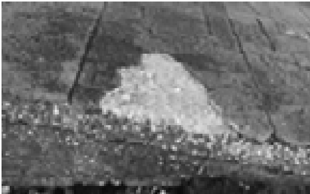
FIGURE 56. View of deterioration on ramp to small boat-room door. (T. Jones, NPS, 2005)
