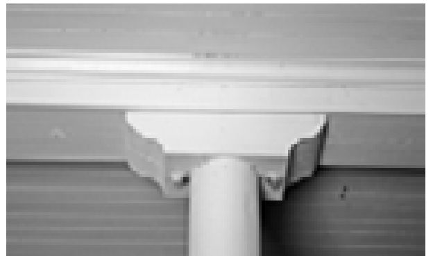
FIGURE 125. View of header and top of post in Room 107. (T. Jones, NPS, 2005)
