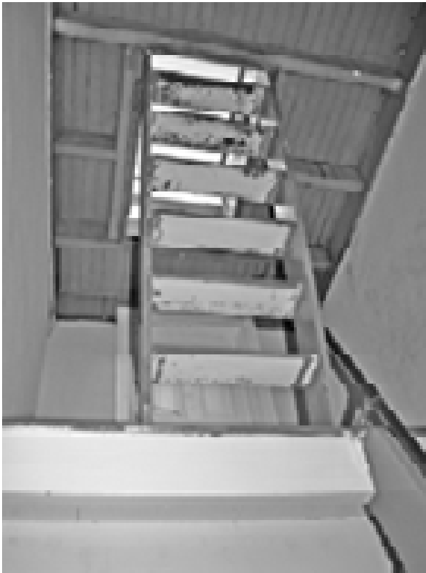
FIGURE 130. View from Room 200 of attic landing and stairs to watch room. (T. Jones, NPS, 2005)
