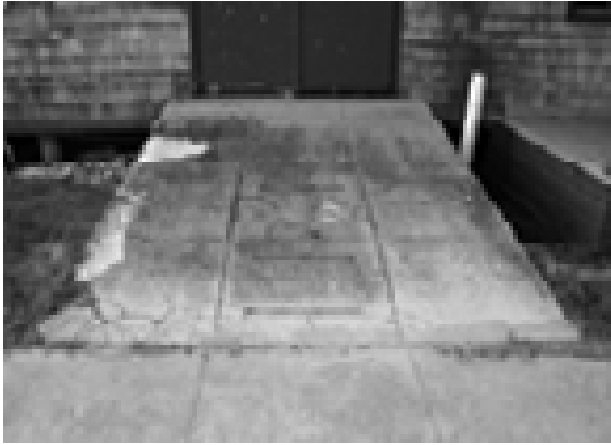
FIGURE 55. View of ramp to smaller boat room door on northwest side of building. (T. Jones, NPS, 2005)
