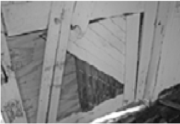
FIGURE 84. View of damage to lower panel of leaf of Boat Room door D-5. (T. Jones, NPS, 2005)
