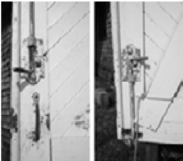
FIGURE 81. View of typical upper (left) and lower (right) sliding bolts on boat room doors. (T. Jones, NPS, 2005)
